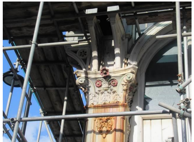
Rust staining and surface corrosion to column head and upper capital
