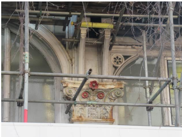
Corrosion and surface pitting to column capitals
