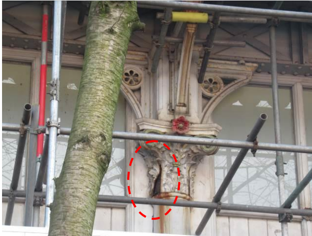
Isolated loss of part to column capital
