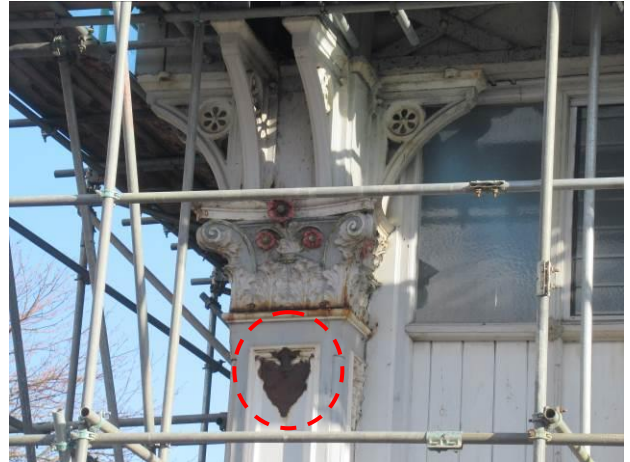
Missing decorative crest to the upper portion of the rear lefthand corner column
