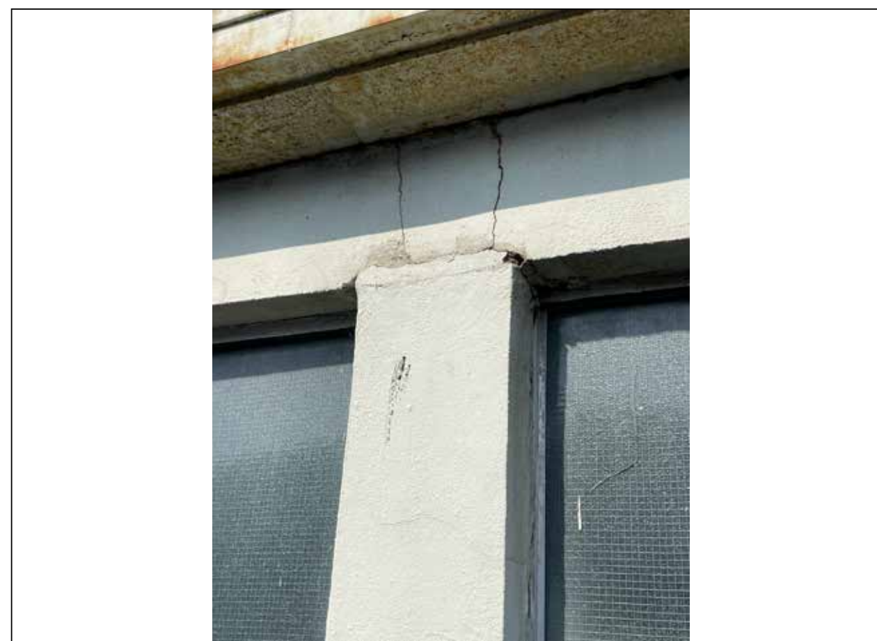
Image 22: Detail of exterior wall in degraded condition.
