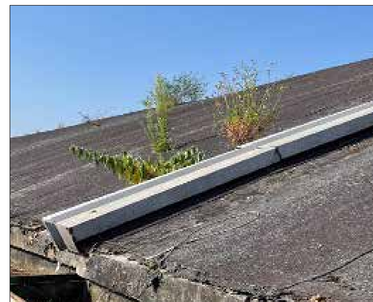
Image 18: Contemporary photograph showing poor condition of roof covering.
