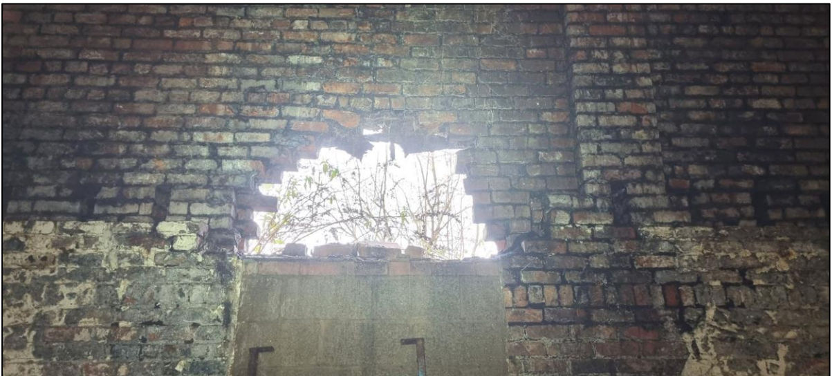
Plate 20: A large hole in the rear wall provided unfettered potential access to the internal space.
