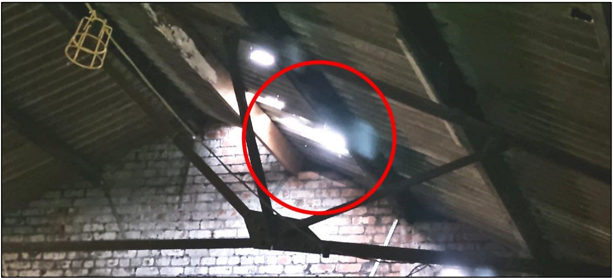
Plate 19: Damaged roofing sheets left a hole in the east facing pitch allowed access to the internal space.
