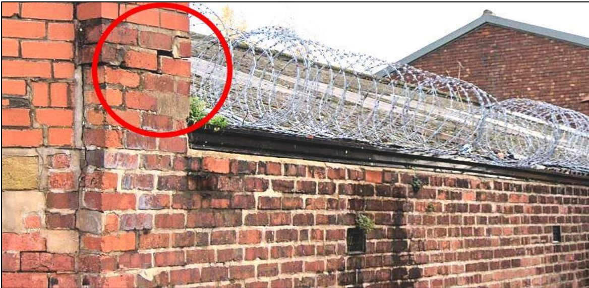
Plate 15: Shallow area of missing mortar in the brickwork was present but were found not to lead to internal crevices or considered to have any roosting potential.
