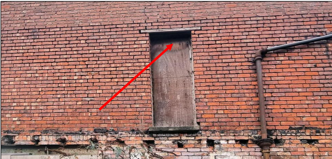
Plate 13: Gaps around previously boarded up doors and windows allowed potential access to the internal space.
