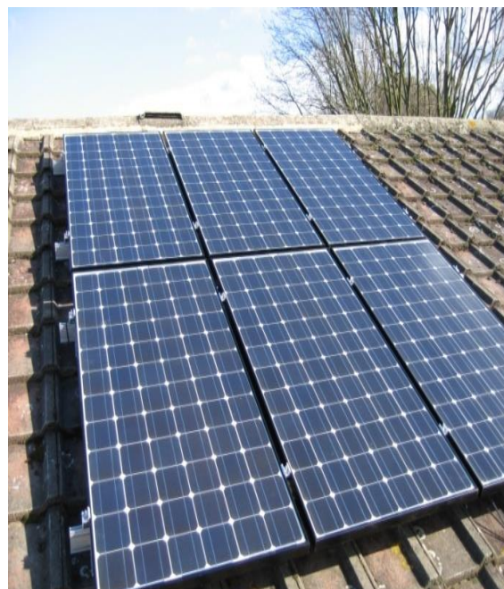
Figure 5 - Photovoltaic array on a pitched roof
