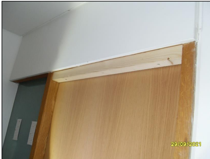
PHOTO 07 – Internal, poorly installed fire door
