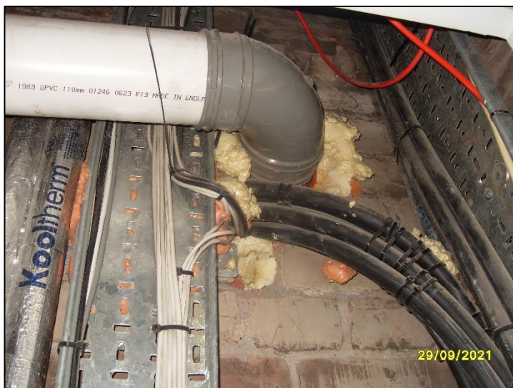
PHOTO 11 – Internal, concealed poorly fire stopped penetration
