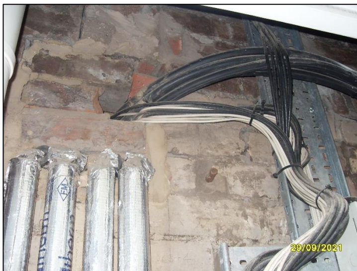
PHOTO 12 – Internal, concealed poorly fire stopped penetration
