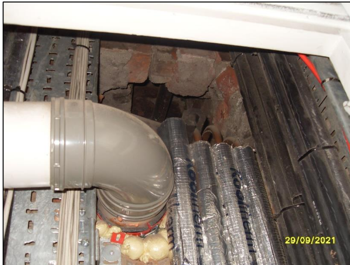
PHOTO 10 – Internal, concealed poorly fire stopped penetration
