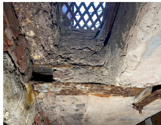
Figure 4: Corroded steel beams, deteriorated concrete soffit, and original ceiling light.
