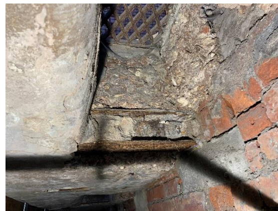
Figure 6: Corroded steel beams, deteriorated concrete soffit, and original ceiling light.
