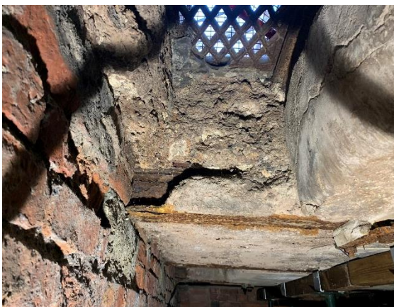
Figure 3: Corroded steel beams, deteriorated concrete soffit, and original ceiling light.
