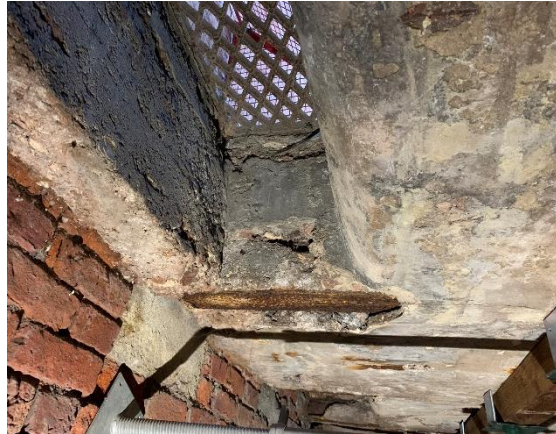
Figure 2: Corroded steel beams, deteriorated concrete soffit, and original ceiling light.
