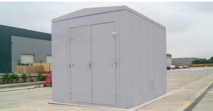
Example Of Proposed GRP Housing Enclosure to Plantroom
