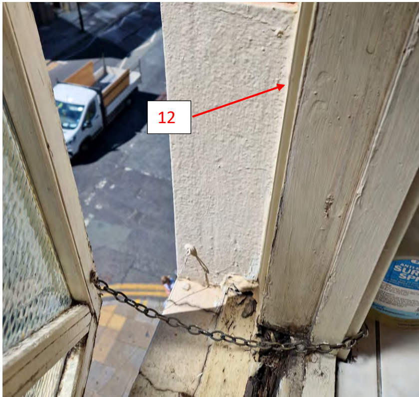
Figure 10: sample location 12 (upper window W8-LG)
