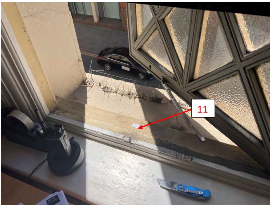
Figure 9: sample location 11 (upper window W11-LG)
