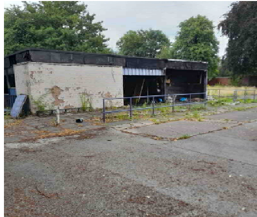
Photograph 5: Derelict smaller building towards the centre of site.
