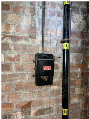
Walsall fuse unit (presume ACMs)
