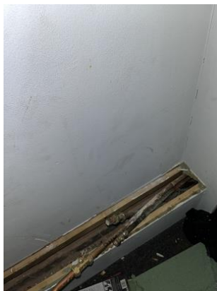
Low level timber boxing to uninsulated pipework
