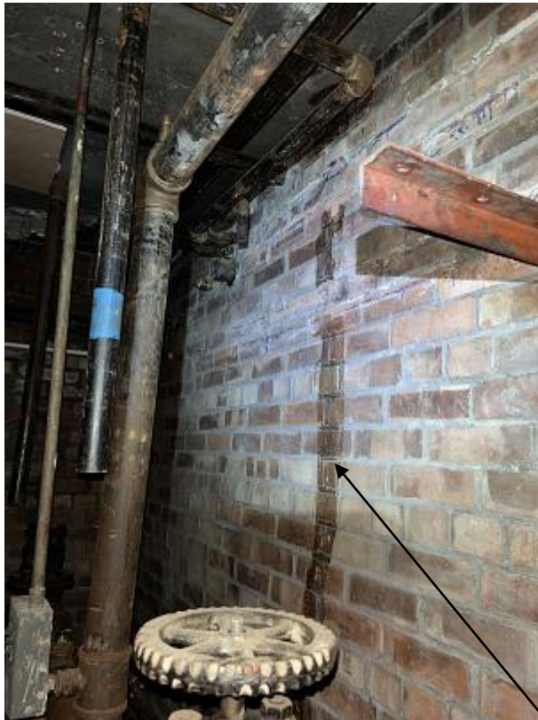
Enclosure glue and duct tape
