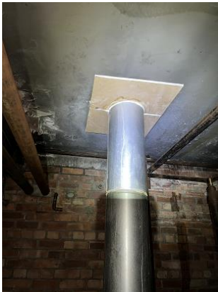
Plasterboard around flue by ceiling penetration
