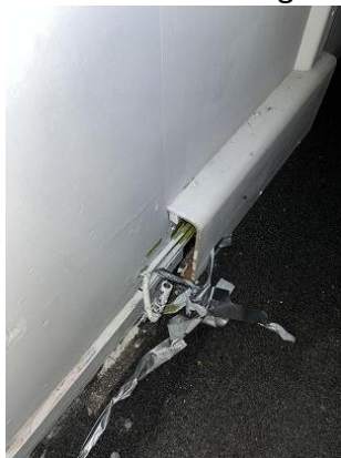
Timber boxing to low level pipework
