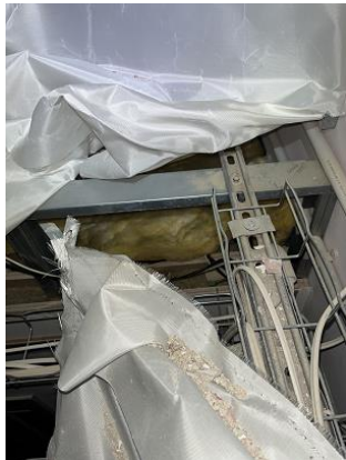
Textile fire breaks (2013) in roof void
