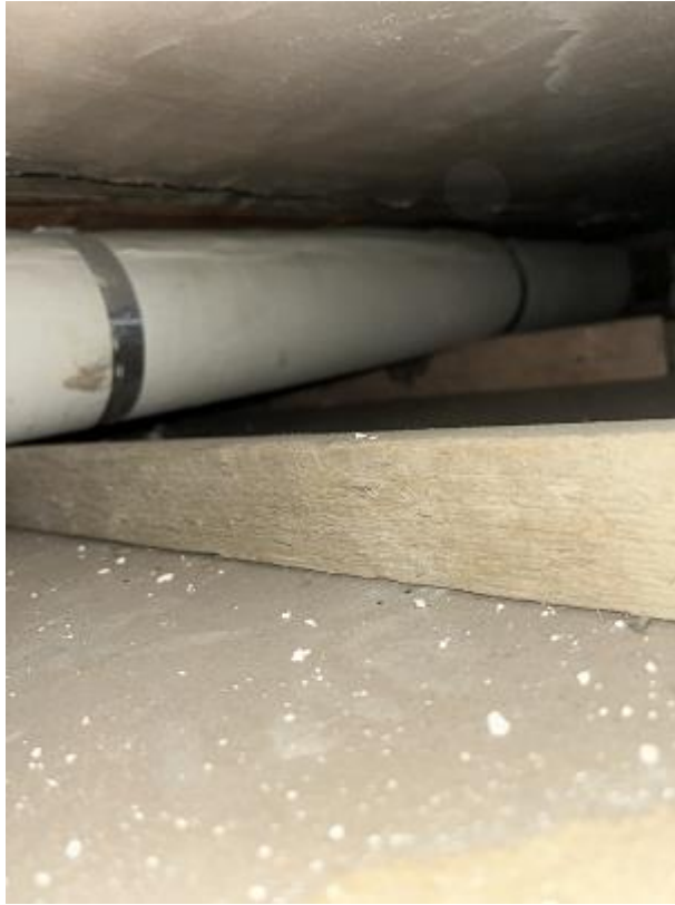
Non-asbestos pipe insulation
