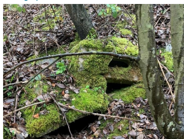
Photograph P02: Hollows within embankment
