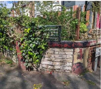
Conditions of the front wall and fencing after removing the overgrown bushes
