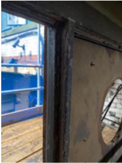
Figure 5: WP.0.07 Internal (Credit Fairhurst 2022)
