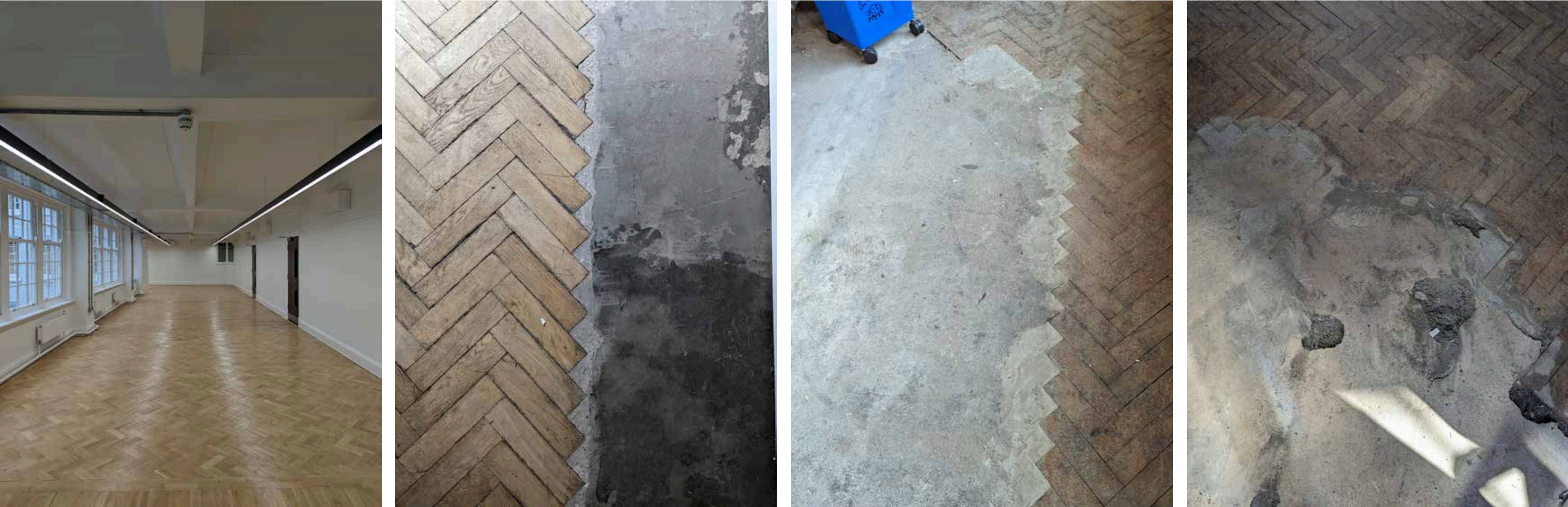
Above - scale of existing parquet to different areas around the building ranging from usable to hazardous.
