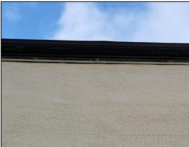
Photograph 3 showing a gap at the soffit
