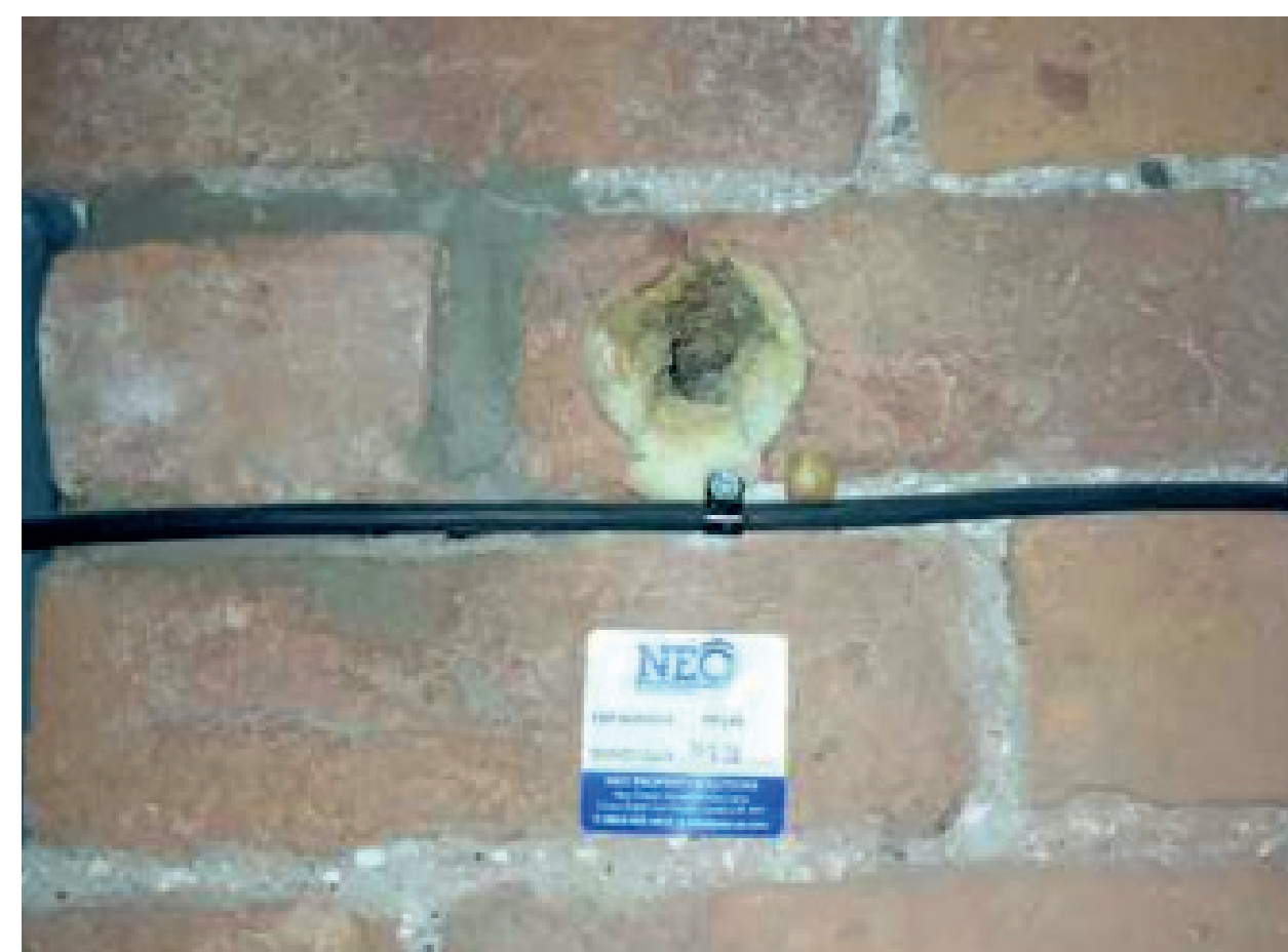
Example of isolated brick requiring a mortar repair
