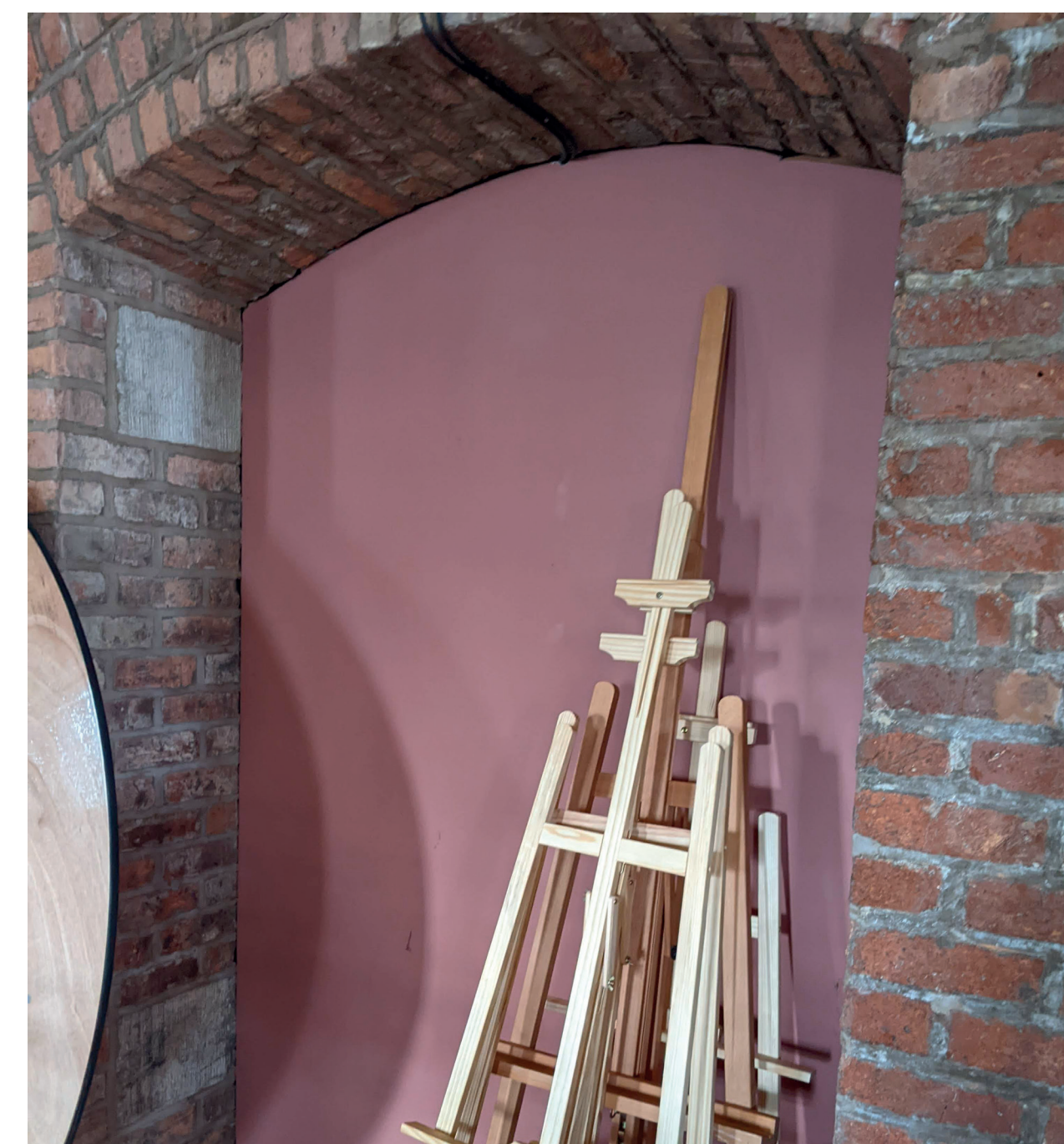
Example of an existing opening within masonry wall. This partition is not sufficiently fire rated and therefore we will upgrade this. Refer to drawings P(110), P(122) and P(123) for locations.
