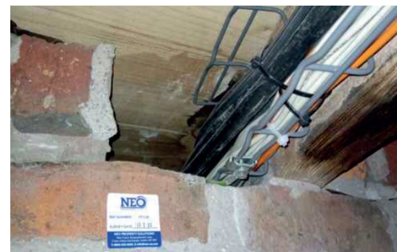
Example photos of localised areas of missing or damaged brickwork to be repaired prior to standard fire stopping details being carried out.
