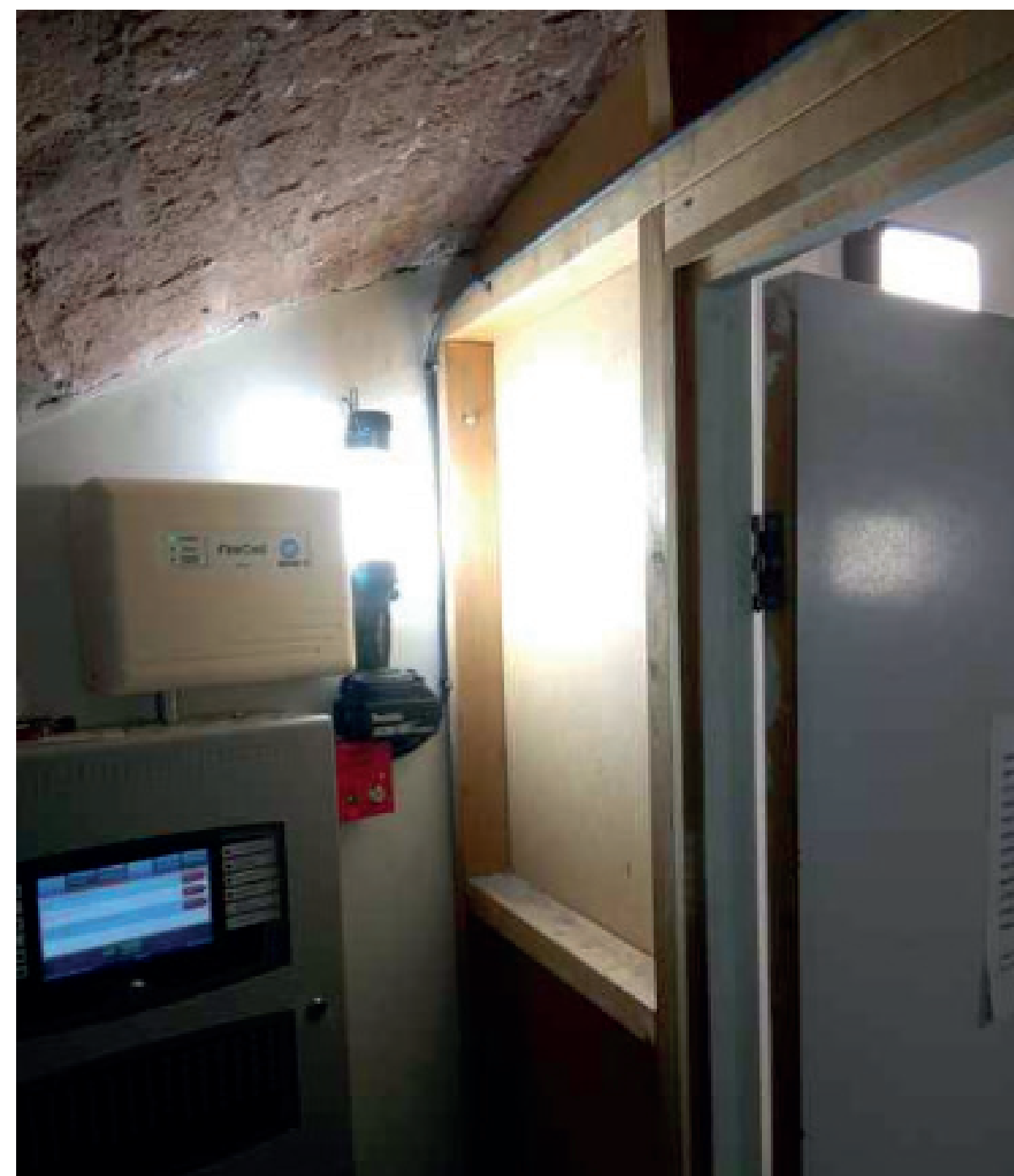
Example of a partition and door which are not fire rated. These will be carefully taken down and a fire rated equivalent reinstated. All fixings will be into the mortar joints of the surrounding brickwork only.
