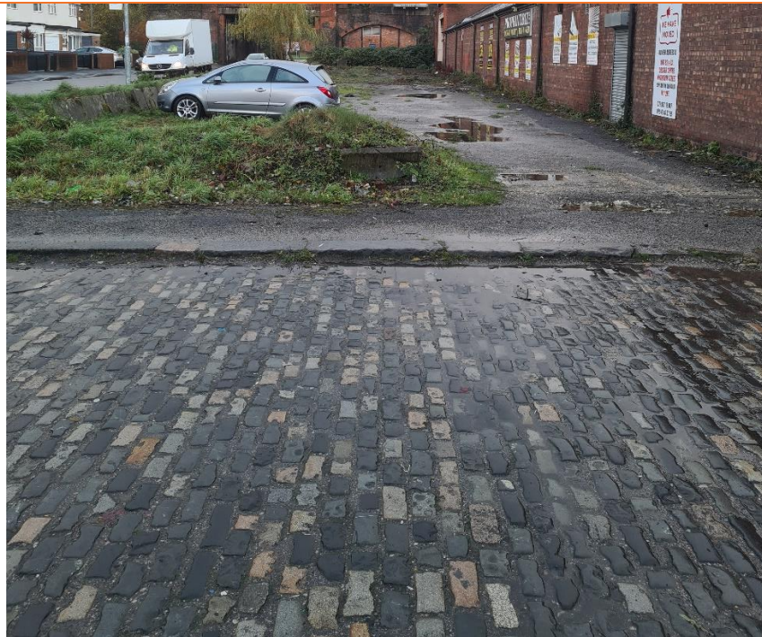
PLATE 2 COBBLES WITH COAL TAR SEALANT DURING E3P 2021 INVESTIGATION
