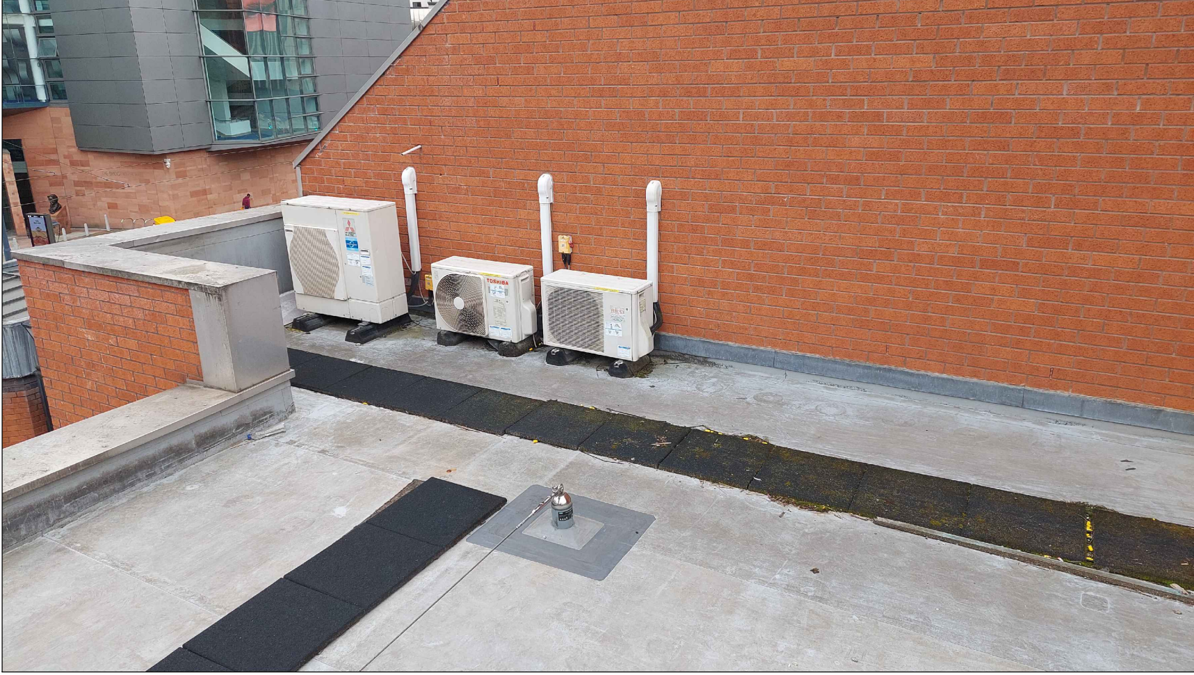
PHOTO 8 – EXISTING 3NO. CONDENSERS SERVING FIRST FLOOR OFFICES.
