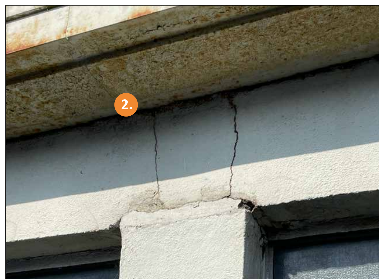
Photo Showing example of concrete damage
