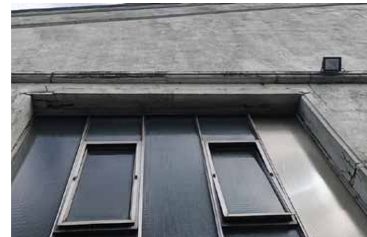
Existing replacement plastic panel (right-hand side).
