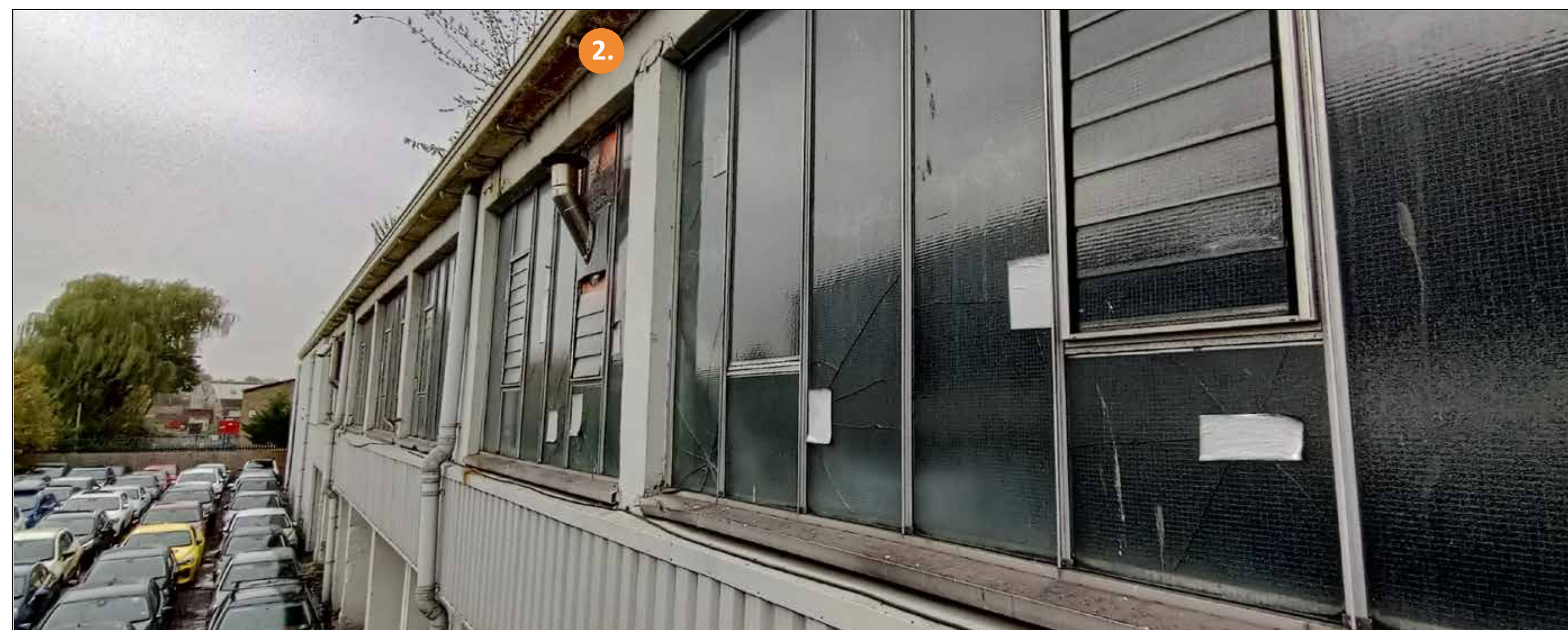
Photo Showing example damage to the north east facade
