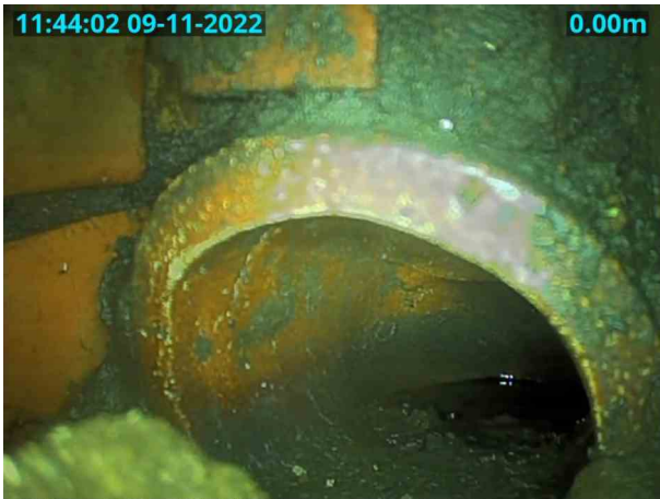
A PIPEX_64e917a8-7065-458f-a29d-cb9614f4c08a_20221126_ 105820_790.jpg, 00:00:18, 0.50 m Survey abandoned, DEBRIS
