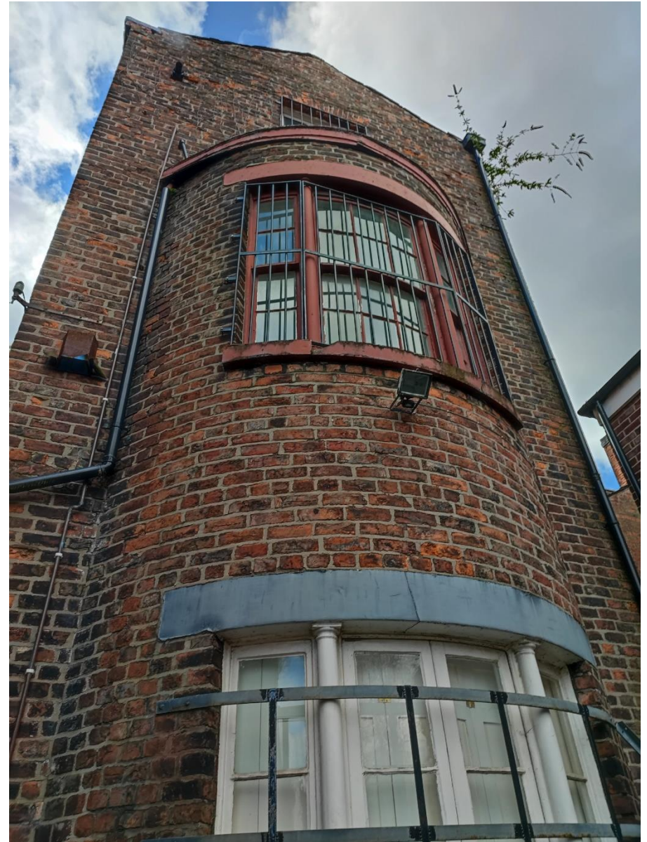
Figure 06 – Close up view Southwest towards rear windows Metal security bars to be removed. Windows to make good or like to like replacement where required.
