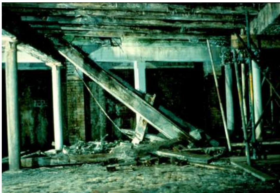
The interior of the 1830 Warehouse basement showing collapsed ceiling timbers and general dereliction
