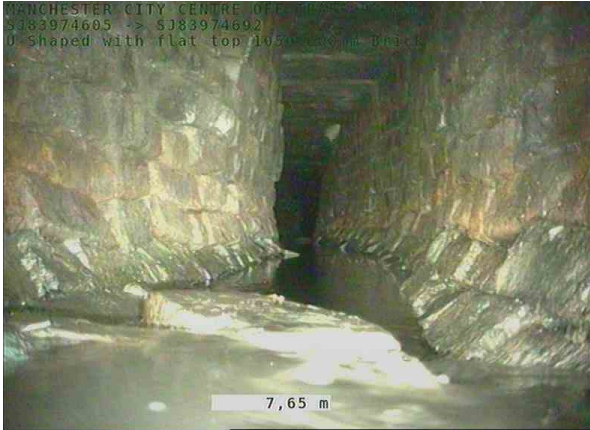
SJ83974605X_14a4666f-e670-42a3-990a-5f2f6a004e00_20180925_211438_410.jpg, 00:00:56, 6.18 m Settled deposits, hard or compacted, 15% cross-sectional area loss
