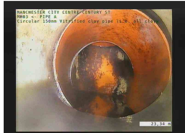
PIPE AX_0e5fd09a-17f5-49d6-8061-8ff7978b154d_20180919_120755_130.jpg, 00:03:04, 23.34 m Joint displaced, large
