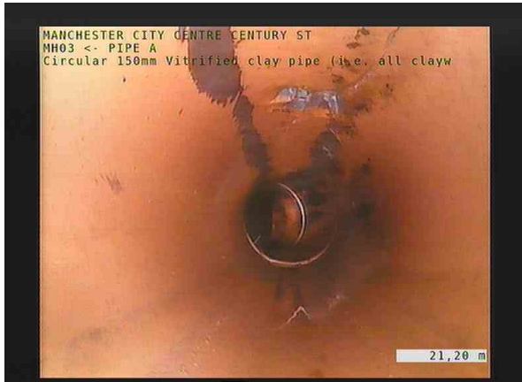
PIPE AX_c69fb965-b39e-4ee7-b7d1-dbf41f212de9_20180919_120705_047.jpg, 00:02:33, 21.20 m Hole in drain or sewer at 12 o'clock
