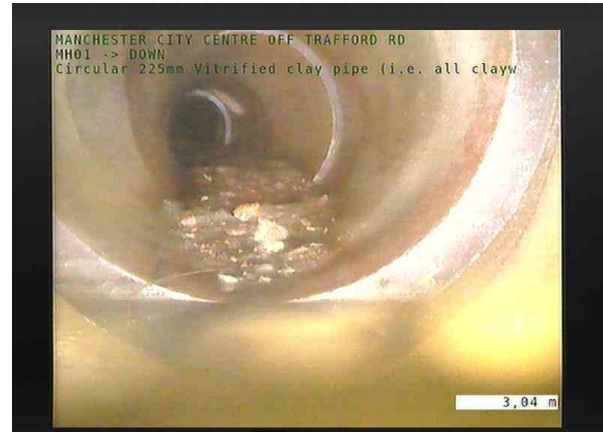
MH01X_f148549a-2cab-4964-9756-ad63c6ee8c38_20180919_105106_079.jpg, 00:02:32, 3.04 m Fracture, circumferential at joint from 6 o'clock to 7 o'clock
