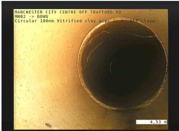
MH02X_332de3c9-d6b1-4ed2-be62-5121e2c691b1_20180919_105840_365.jpg, 00:00:31, 4.53 m Fracture, circumferential at joint from 10 o'clock to 2 o'clock
