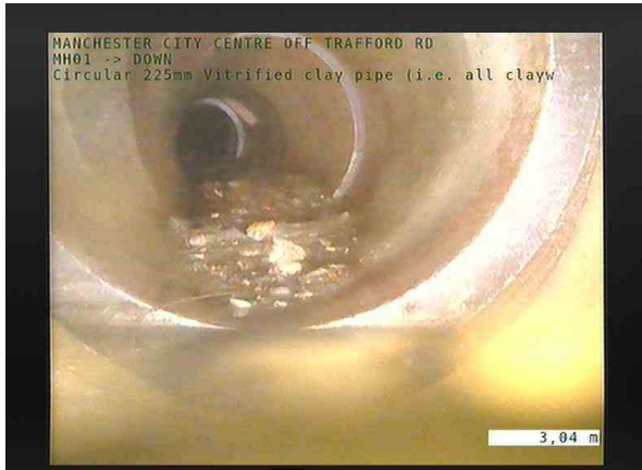
MH01X_fa4ee0e4-04f6-48b5-a3ee-063efc016c2a_20180919_105103_342.jpg, 00:02:29, 3.03 m Joint displaced, large
