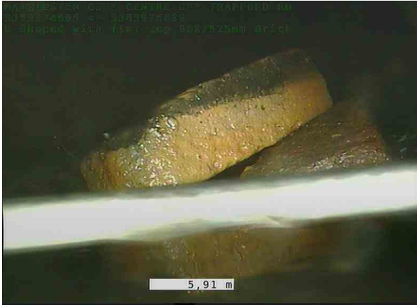
SJ83975609X_45d3f61b-c28b-43cc-8abd-9c57f23fda29_20180925_213249_967.jpg, 00:03:06, 5.91 m Settled deposits, hard or compacted, 30% cross-sectional area loss
