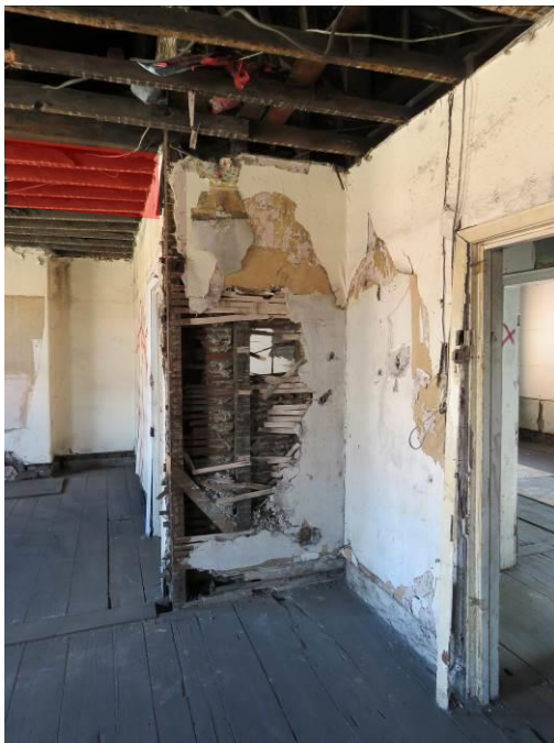
Figure 152 – Looking east towards 2F03 from 2F02, showing the consented removal of dividing wall, and unconsented removal of downstand (shaded red) and lath and plaster ceiling.
