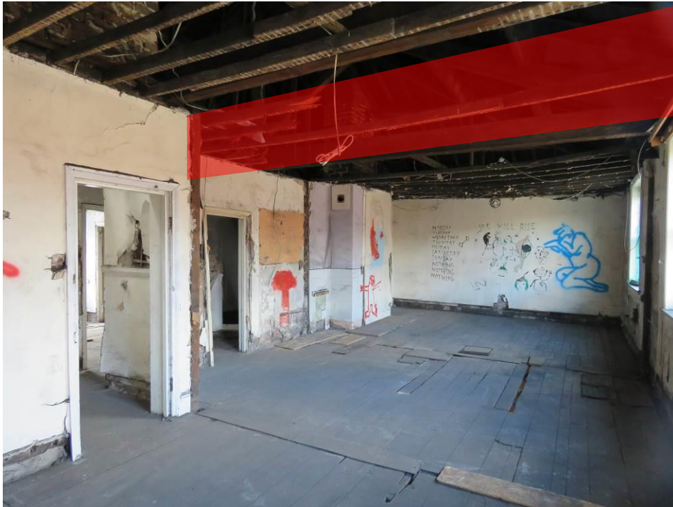
Figure 146 – Looking west from 2F03, into 2F02 and 2F01, showing the consented removal of walls, but the unconsented removal of the downstand beam (shaded red), lath and plaster ceilings and skirtings.
