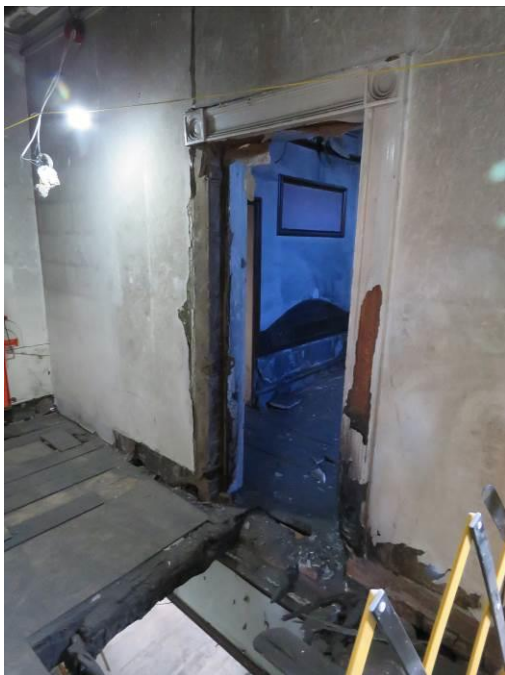
Figure 140 – Looking across corridor 1F07 towards the door opening into 1F08, which is inaccessible due to fire damage to the floor in front. Note the original panelled door and the left architrave is now missing.
