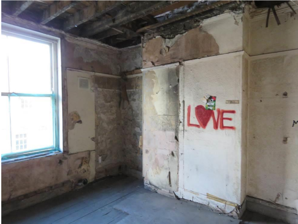
Figure 130 – Looking into 1F03, showing the consented removal of modern bathroom en-suite to the corner alcove, and unauthorised removal of original lath and plaster ceiling, cornice and skirtings.
