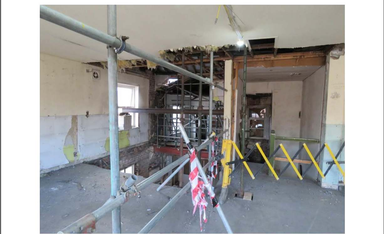
Figure 93 – Looking south from 2F14 into the collapsed area of the building (2F17). The stairs (2F16) can be seen to the right.
