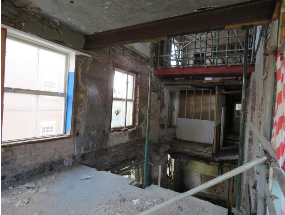
Figure 88 – The collapsed area of the first floor level (1F14) looking into 1F16.
