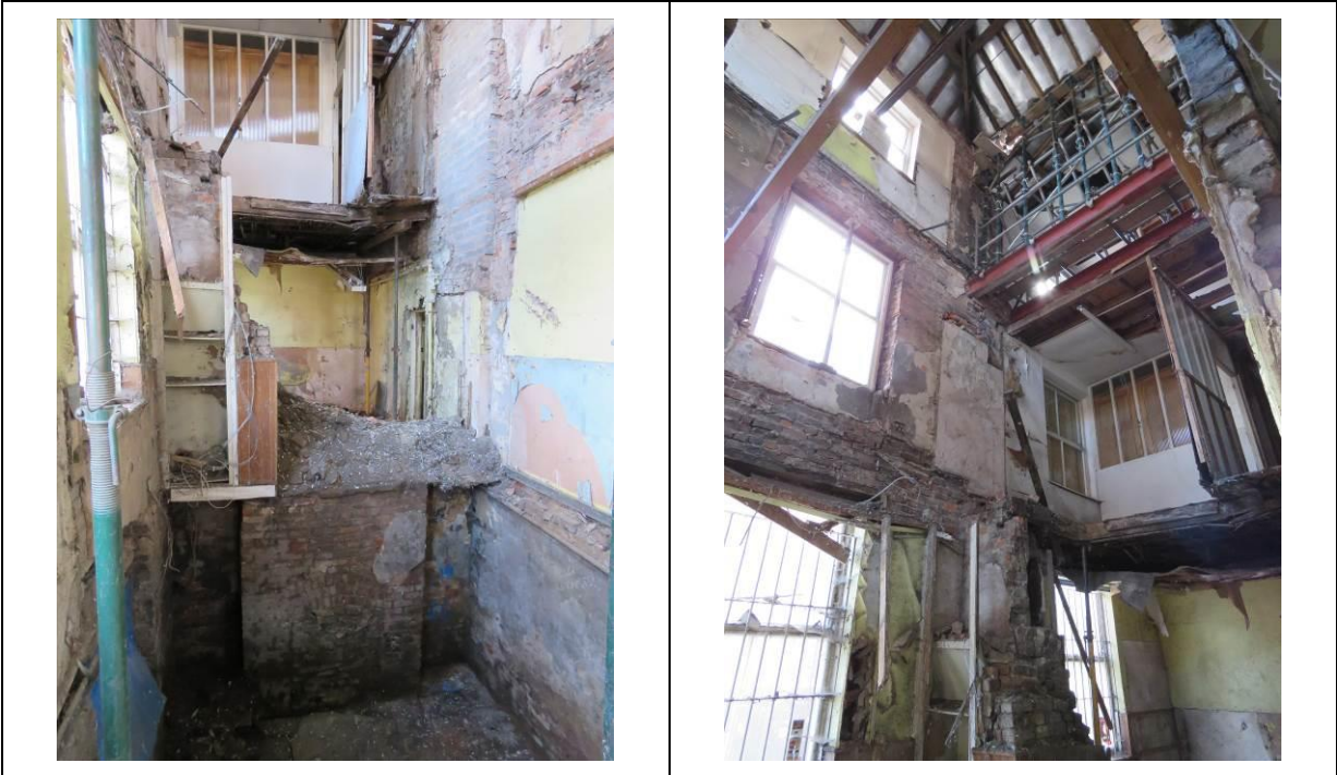
Figure 78 – Looking towards the southern end of the area of collapse (GF13).
