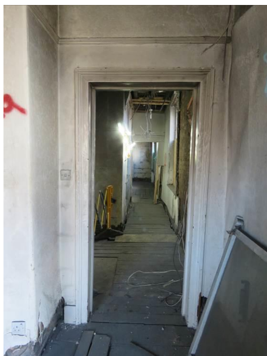
Figure 128 – A closer view of the location of the missing original panelled door into 1F01.
