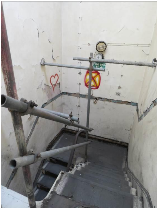
Figure 164 – Looking down the original staircase (2F04), showing the removed original balustrading/handrails and dado rail.
