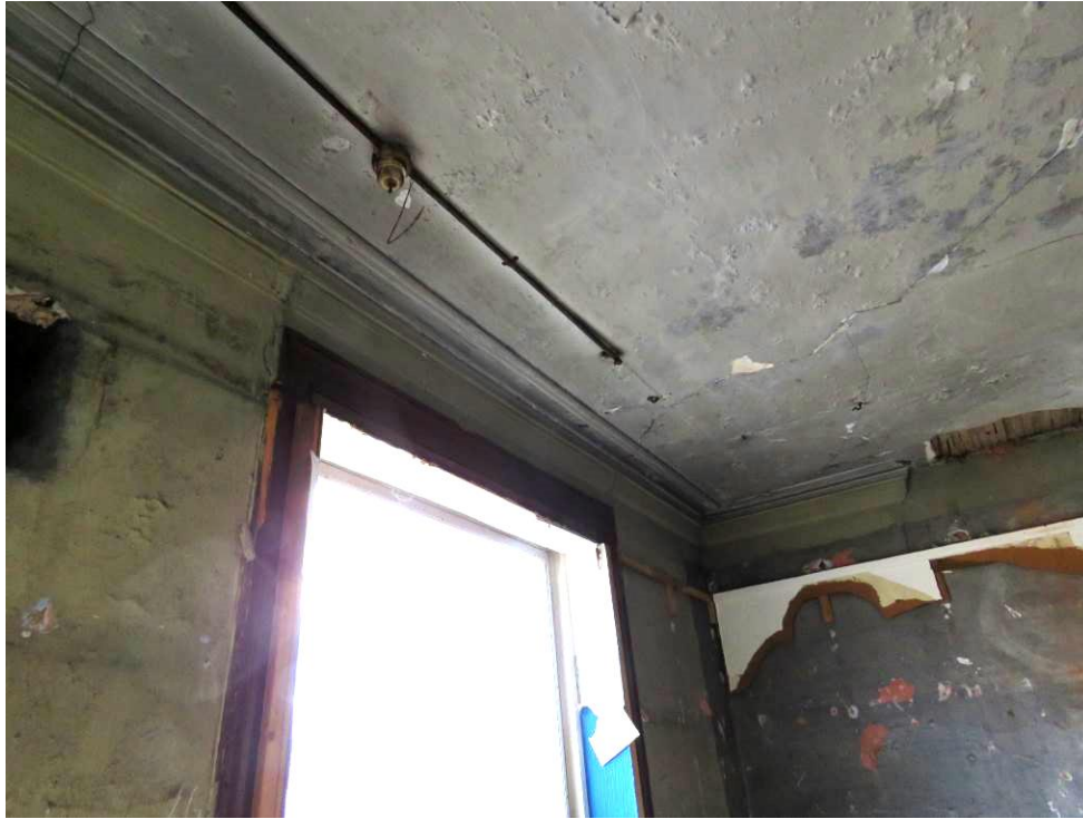
Figure 90b – A length of newly uncovered original moulded timber window surround and plaster cornice above one of the windows in 1F14
