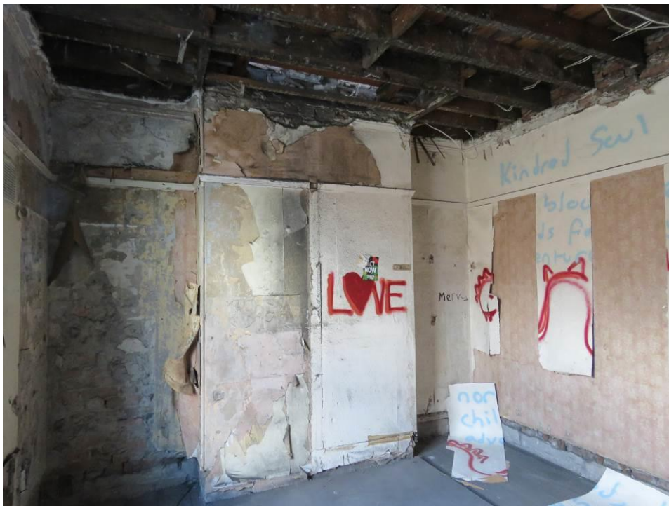
Figure 131 – The east elevation of 1F03, showing the consented removal of modern bathroom en-suite to the corner alcove (left) and unauthorised removal of original lath and plaster ceiling, cornice and skirtings
