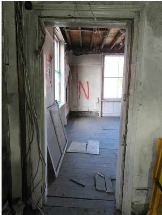
Figure 145 – The corridor side of the entrance into 1F01, showing the missing panelled door.
