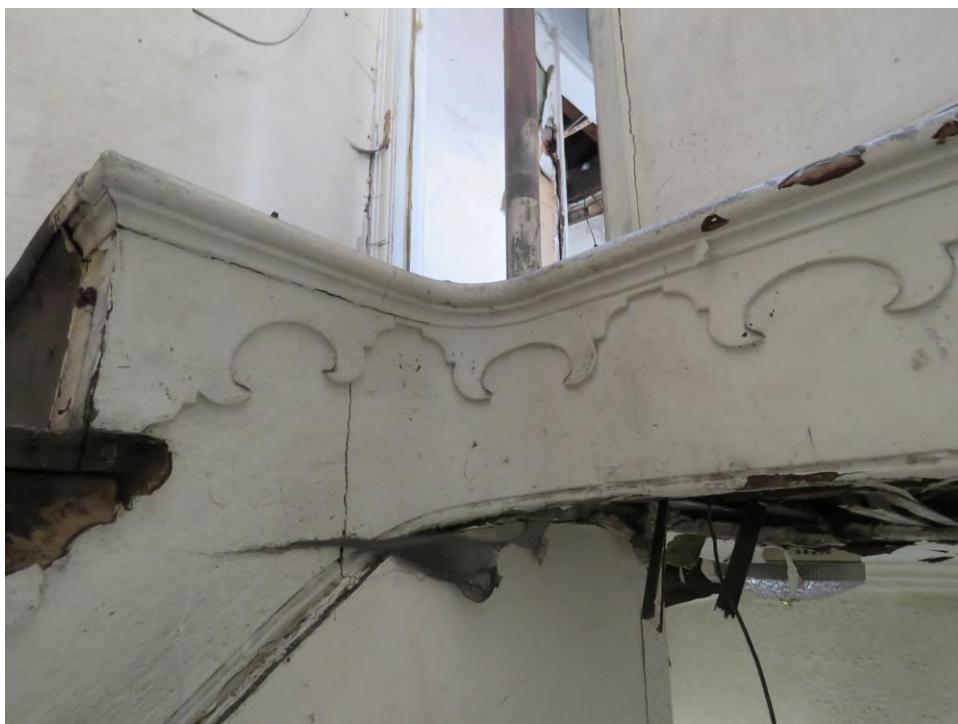
Figure 165 – Detail of the original cut string carved decoration to 2F04.
