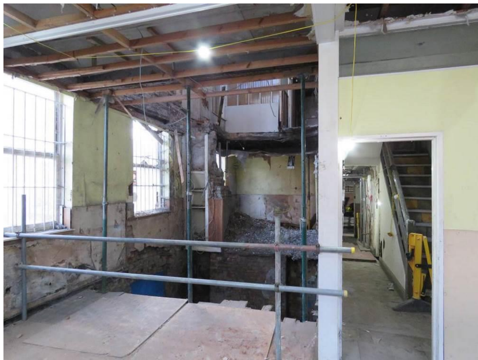
Figure 76 – Looking south through the eastern part of GF13 showing the large area of collapse from second to basement floor levels.
