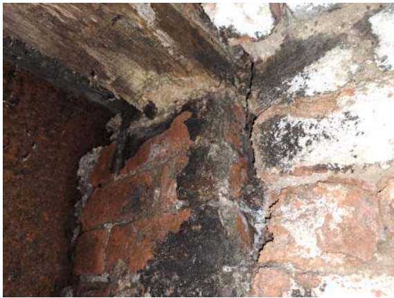
B15: JOINT BETWEEN SKINS OF MASONRY ADJACENT TO PAVEMENT LIGHT HAS OPENED UP ON THE WOOLLAM PLACE ELEVATION OF ROOM B07.
