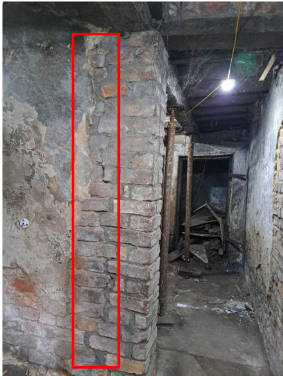
B25: VERTICAL CRACK IN WALL ADJACENT TO STAIRS IN ROOM B09 AT BEARING POINT FOR TIMBER BEAM ABOVE.
