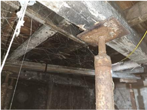
B21: HISTORIC PROPPING TO TIMBER BEAMS SUPPORTING THE GROUND FLOOR OVER ROOM B10. THE BEAMS AND JOISTS IN THIS AREA APPEAR TO BE IN VARIABLE CONDITION.
