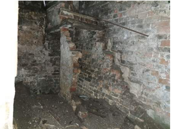
B18: COLLAPSED STAIRS FROM BASEMENT TO GROUND FLOOR WITHIN INACCESSIBLE PART OF BASEMENT TO 123 LIVERPOOL ROAD. VIEWED FROM DOOR OPENING FROM ROOM B10.
