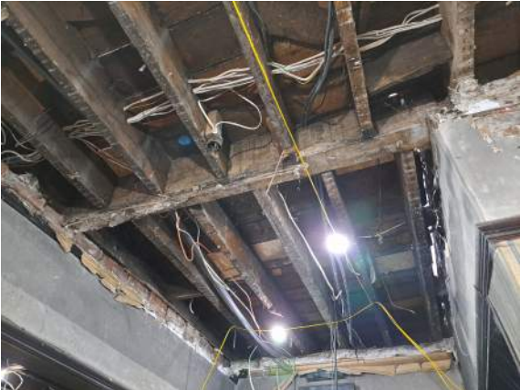
G02: TIMBER BEAM ABOVE ROOM G02. HOLES HAVE BEEN FORMED THROUGH THE BEAM TO ALLOW FOR SERVICES.
