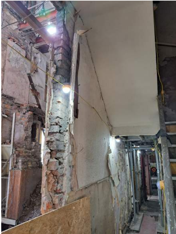
G11: VISIBLE BOWING OF LOAD-BEARING MASONRY WALL ADJACENT TO STAIRS IN ROOM G06. RESTRAINT TO WALLS FROM FLOORS HAS BEEN LOST DUE TO ADJACENT COLLAPSE WITHIN ROOM G05.
