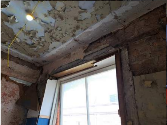
118: THE LINTEL AND MASONRY OVER A WINDOW OPENING ON THE LIVERPOOL ROAD ELEVATION OF ROOM 107 APPEARS TO HAVE DIPPED AT ONE END.
