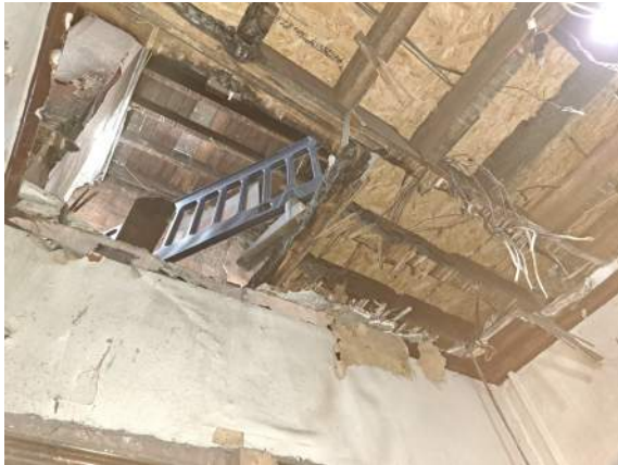
G01: AFIRE DAMAGE AND LOSS OF SECTION TO 1ST FLOOR TIMBER JOISTS AROUND RISER OPENING ADJACENT TO BAR ABOVE ROOM G02.
