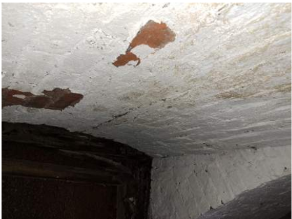
B13: HORIZONTAL CRACK AT THE CROWN OF A MASONRY ARCH OVER A PAVEMENT LIGHT WITHIN ROOM B07.
