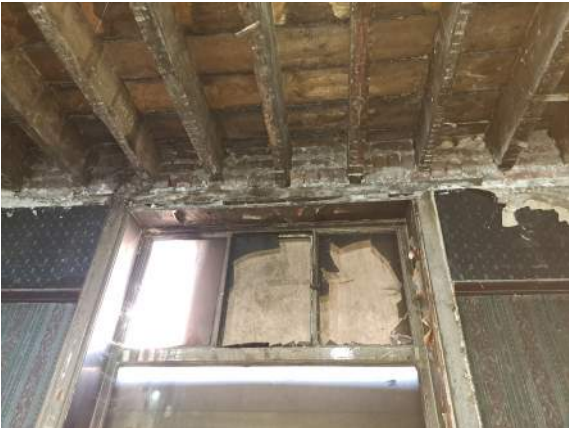
G05: SIGNS OF DECAY TO TIMBER LINTEL OVER WINDOW OPENING ON LIVERPOOL ROAD ELEVATION OF ROOM G02.
