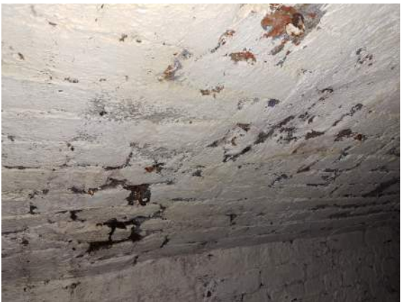
B17: LOCALISED DISPLACEMENT OF MASONRY ON UNDERSIDE OF VAULTED CEILING WITHIN ROOM B07.
