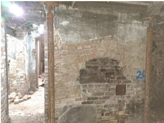
B20: VERTICAL CRACK THROUGH MASONRY CHIMNEY BREAST IN ROOM B10.
