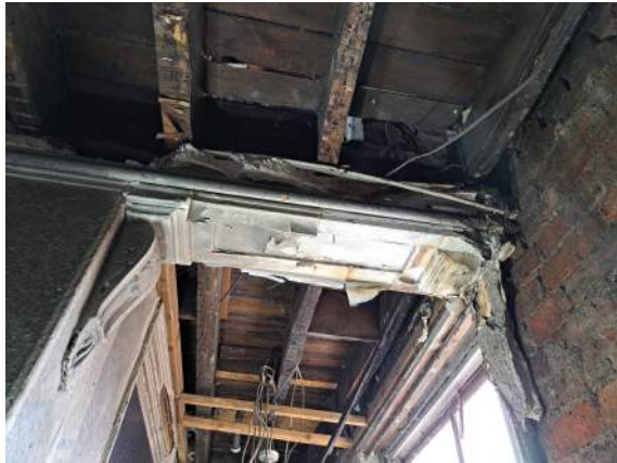
106: TIE ROD TO UNDERSIDE OF 2ND FLOOR HAS BEEN CONCEALED WITHIN CORNICE OVER ROOM 104. SIGNS OF CORROSION WHERE ROD PASSES THROUGH EXTERNAL WALL ON WOOLLAM PLACE.
