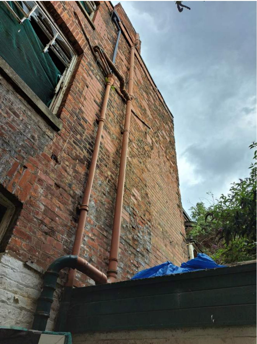
E03: VISIBILITY OF SOUTH ELEVATION TO 123 AND 125 LIVERPOOL ROAD ABOVE REAR EXTENSION IS LIMITED DUE TO SIGNIFICANT VEGETATION GROWTH. EVIDENCE OF NUMEROUS HISTORIC REPAIRS/AREAS OF RE-BUILDING.
