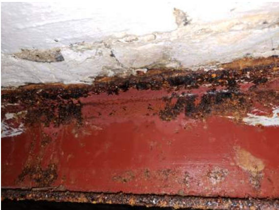
B12: CORROSION OF THE REMEDIAL STEEL BEAMS SUPPORTING THE CROWN OF THE VAULTED CEILING OVER ROOM B07.
