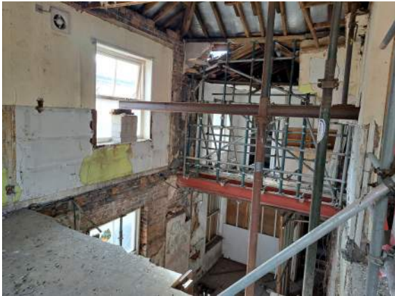
217: VIEW OF COLLAPSE AT 2ND FLOOR. RENAISSANCE HAVE DESIGNED TEMPORARY PROPPING TO SUPPORT SECTION OF ROOF ON LINE OF COLLAPSED WALL AS PART OF INITIAL MAKING SAFE WORKS. PROPPING HAS ALSO BEEN INSTALLED HISTORICALLY DESIGNED BY OTHERS.
