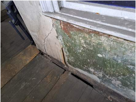
108: CRACKING UNDER INTERNAL WINDOW OPENING SEPARATING ROOM 104 FROM INACCESSIBLE BATHROOM.
