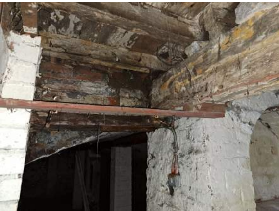
B05: TIMBER BEAM SUPPORTED BY LINTEL OVER DOOR OPENING INTO ROOM B07.
