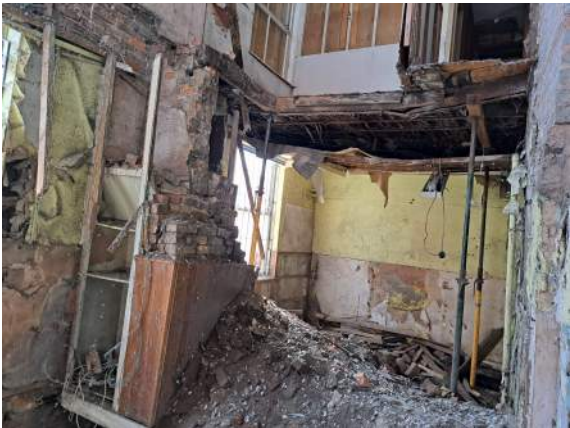
G12: LOAD-BEARING MASONRY WALL AND TIMBER FLOORS AT GROUND, 1ST AND 2ND FLOOR HAVE COLLAPSED. SECTION OF GROUND FLOOR IS INACCESSIBLE TO REAR OF ROOM G05. TEMPORARY PROPS HAVE BEEN INSTALLED TO SUPPORT FAILED TIMBER FLOOR ABOVE.
