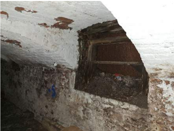
B10: INFILLED PAVEMENT LIGHT WITHIN ROOM B07. THERE ARE SIGNS OF WATER INGRESS THROUGH THE INFILL.
