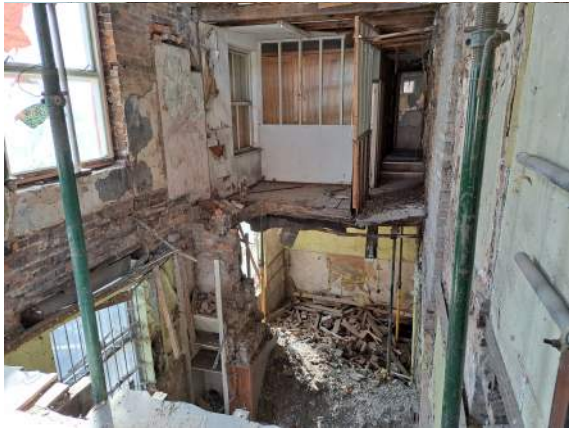
115: 1ST FLOOR HAS COLLAPSED IN ROOM 107. THE PARTITION WALLS WITHIN THE INACCESSIBLE AREA TO THE REAR OF 123 LIVERPOOL ROAD APPEAR TO BE UNSTABLE DUE TO FAILURE OF TIMBER JOISTS BELOW.
