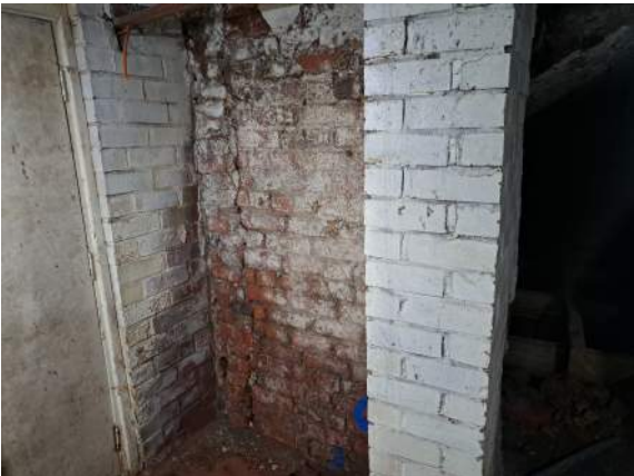
B07: VERTICAL CRACK TO MASONRY WALL BETWEEN ROOMS B06 AND B07.
