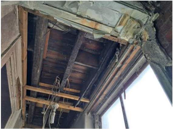
107: TIMBER JOIST OVER ROOM 104 ADJACENT TO EXTERNAL WALL ON WOOLLAM PLACE HAS DECAYED DUE TO WATER INGRESS.
