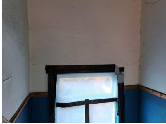
221: MINOR CRACKING OF FINISHES PROPAGATING FROM CORNERS OF WINDOW OPENING ON REAR ELEVATION OF ROOM 207.
