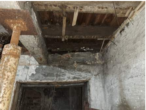
B19: LINTEL OVER DOOR OPENING FROM ROOM B10 TO INACCESSIBLE PART OF BASEMENT TO 123 LIVERPOOL ROAD HAS DEFLECTED AT BEARING POINT OF TIMBER BEAM.
