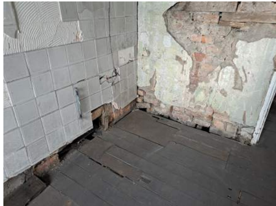
206: DAMAGE TO MASONRY PARTITIONS IN ROOM 204. THE PARTITIONS ARE IN VARIABLE CONDITION THROUGHOUT THE 2ND FLOOR OF 125 LIVERPOOL ROAD.
