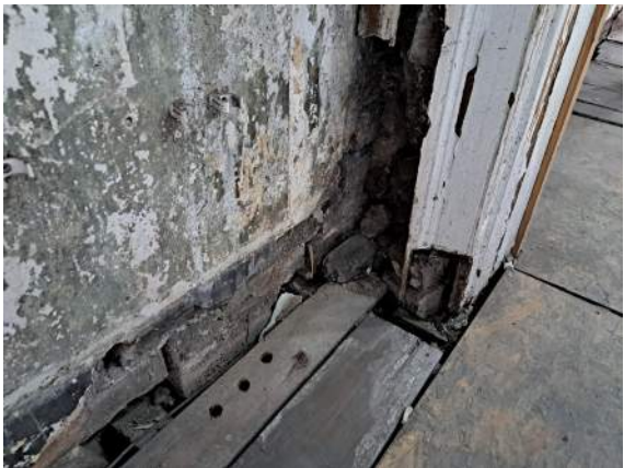
112: BASE OF DOOR FRAME BETWEEN ROOMS 104 AND 105. MAXIMUM HORIZONTAL DEFLECTION OF APPROXIMATELY 80mm OVER HEIGHT OF DOOR FRAME. GAP HAS ALSO OPENED UP BETWEEN TIMBER FLOOR AND EXTERNAL WALL.
