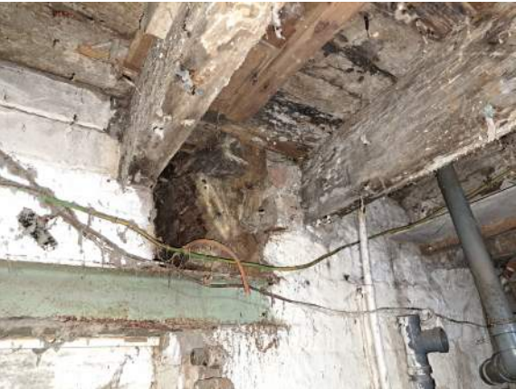
B04: TIMBER ROT AT THE END OF A BEAM SUPPORTING THE GROUND FLOOR OVER ROOM B04 AS VIEWED FROM THE OTHER SIDE OF THE WALL IN ROOM B05.
