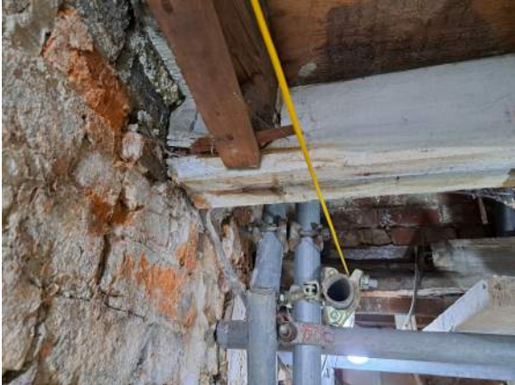
G09: FAILED END BEARING OF TIMBER BEAM SUPPORTING HALF-LANDING OF STAIRS OVER ROOM G06.
