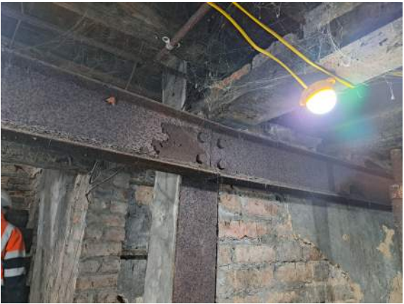
B22: CORROSION OF STEEL COLUMN AND TIE MEMBERS EMBEDDED WITHIN WALL BETWEEN ROOMS B10 AND B11.
