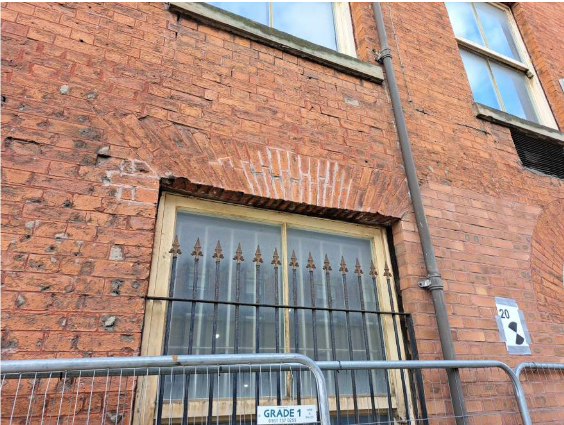
E09: DEFLECTION OF BRICKWORK OVER WINDOW OPENING ON NORTH ELEVATION TO 123 LIVERPOOL ROAD. THE MORTAR JOINTS HAVE BEEN RECENTLY RE-POINTED.
