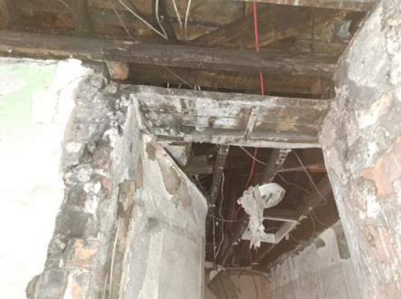
210: TIMBER LINTEL OVER DOOR OPENING BETWEEN ROOMS 202 AND 206 IS DECAYED.
