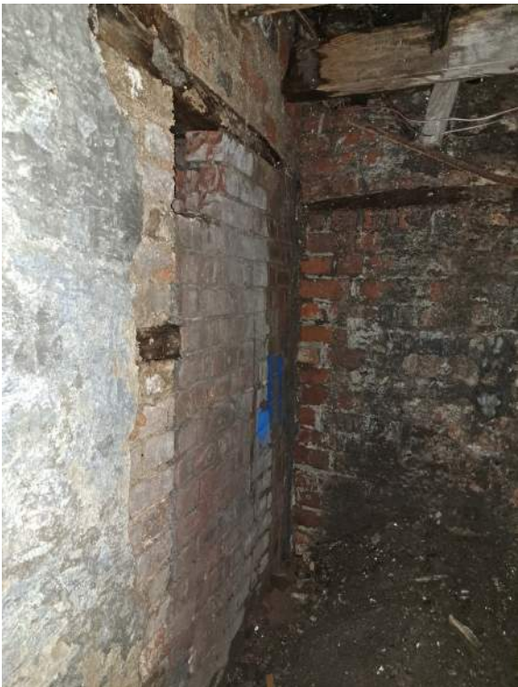
B26: HISTORIC DOOR OPENING INFILLED WITH MASONRY AT END OF CORRIDOR ADJACENT TO STAIRS IN ROOM B09. BUILD-UP OF RUBBLE BEHIND THE INFILL IS VISIBLE.
