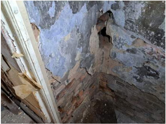
G08: SECTION OF MASONRY MISSING FROM WALL ADJACENT TO STAIRS FROM GROUND FLOOR TO BASEMENT IN ROOM G06.
