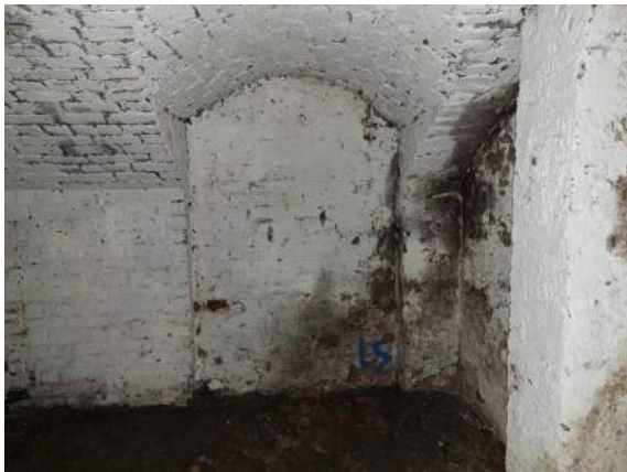
B11: HISTORIC DOOR OPENING INFILLED WITH MASONRY IN THE SOUTH EAST CORNER OF ROOM B07.
