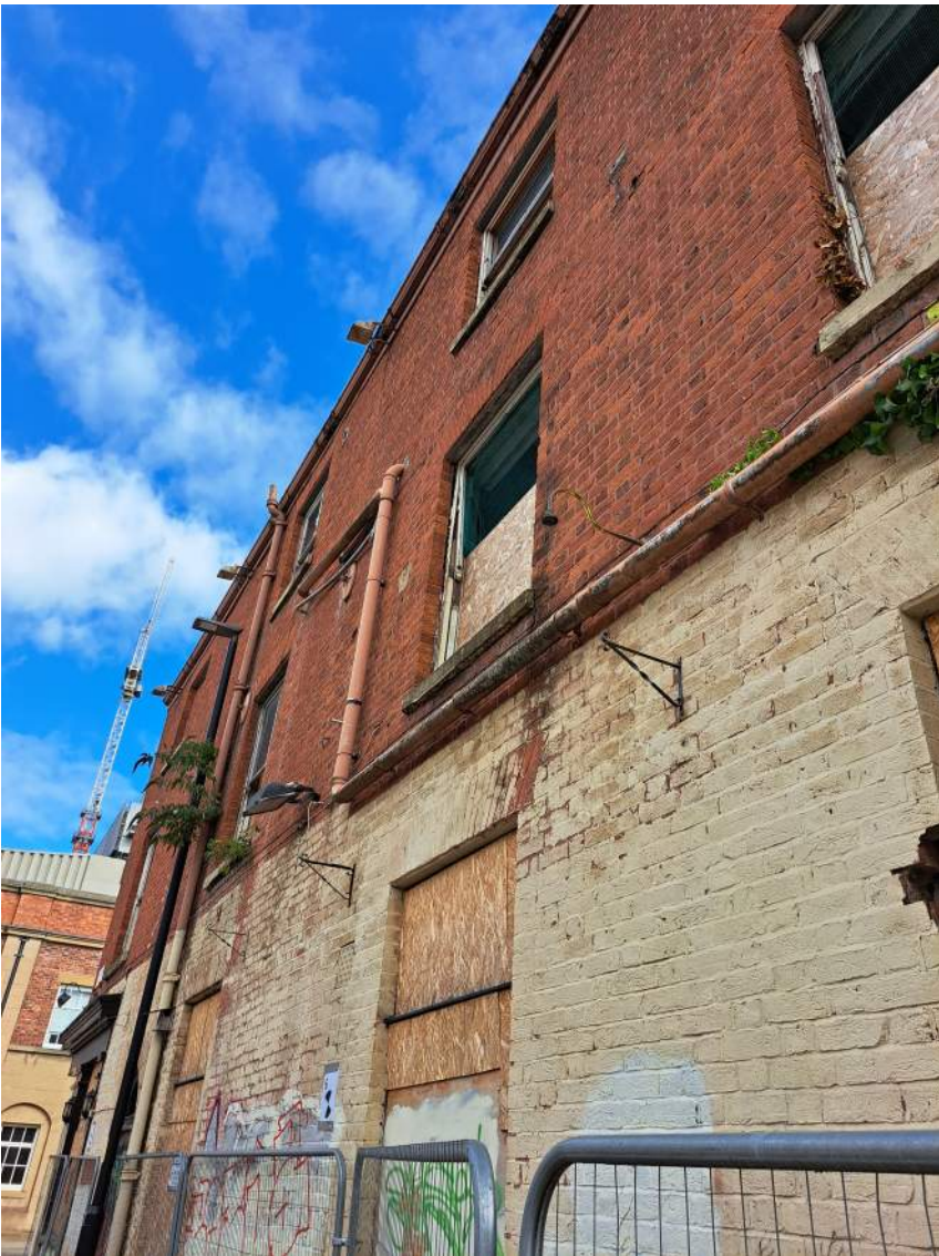
E14: WEST ELEVATION TO 125 LIVERPOOL ROAD. THERE IS A VISIBLE BOW TO THE GABLE WALL AND PATRESS PLATES HAVE BEEN INSTALLED AT 2ND FLOOR. EXTERNAL DRAINAGE IS IN POOR CONDITION.
