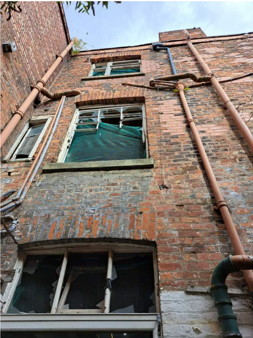
E02: SOUTH ELEVATION TO 125 LIVERPOOL ROAD WITHIN COURTYARD. TIMBER FASCIA AT EAVES LEVEL AND RAINWATER GOODS ARE GENERALLY IN POOR CONDITION.
