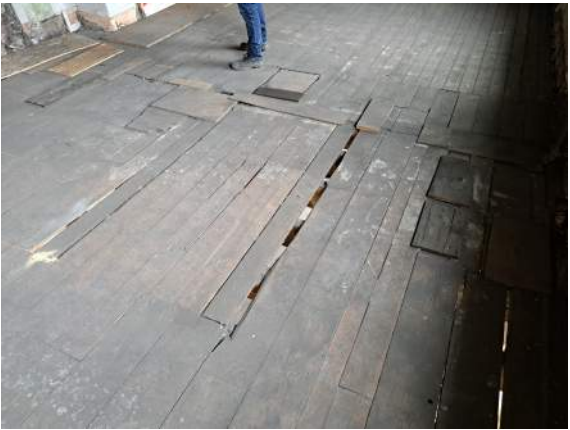
202: FLOOR BOARDS WITHIN ROOM 203 ARE IN VARIABLE CONDITION AND HAVE BEEN SUBJECT TO PATCH REPAIRS.
