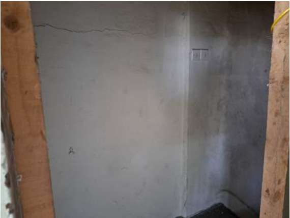
116: HORIZONTAL CRACK ACROSS THE FACE OF THE LOAD-BEARING MASONRY WALL FROM WITHIN THE STAIRS ADJACENT TO THE INACCESSIBLE PART OF ROOM 107.
