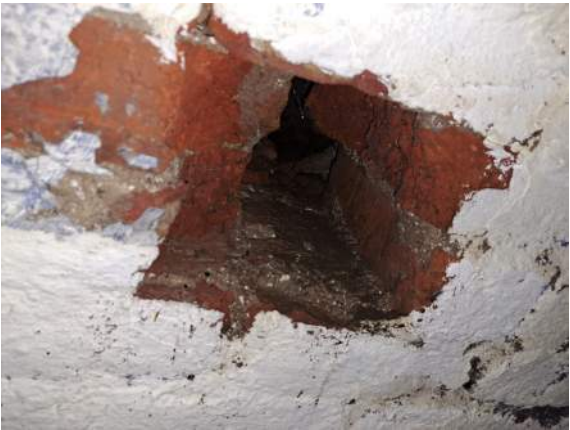
B16: HOLE FORMED THROUGH VAULTED MASONRY ABOVE ROOM B07.
