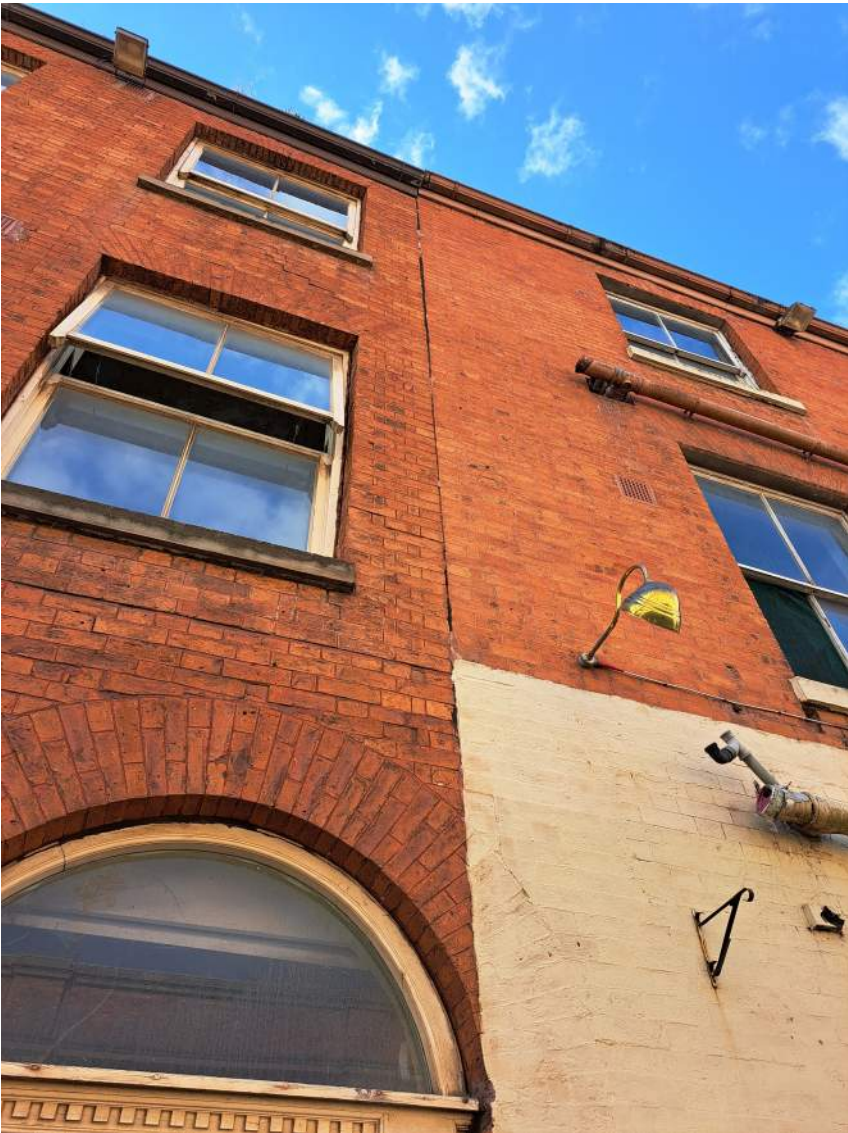
E11: JOINT BETWEEN 123 AND 125 LIVERPOOL ROAD. CRACKING OF MORTAR JOINTS IS VISIBLE BETWEEN THE 1ST AND 2ND FLOOR WINDOWS. EVIDENCE OF MOVEMENT IS APPARENT ABOVE 1ST FLOOR.
