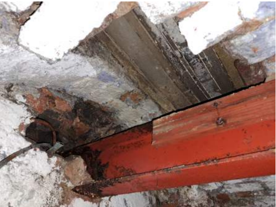
B14: REMEDIAL STEEL BEAM EMBEDDED INTO THE EXTERNAL END WALL OF ROOM B07. CORROSION WAS NOTED AT THE END OF THE BEAM.
