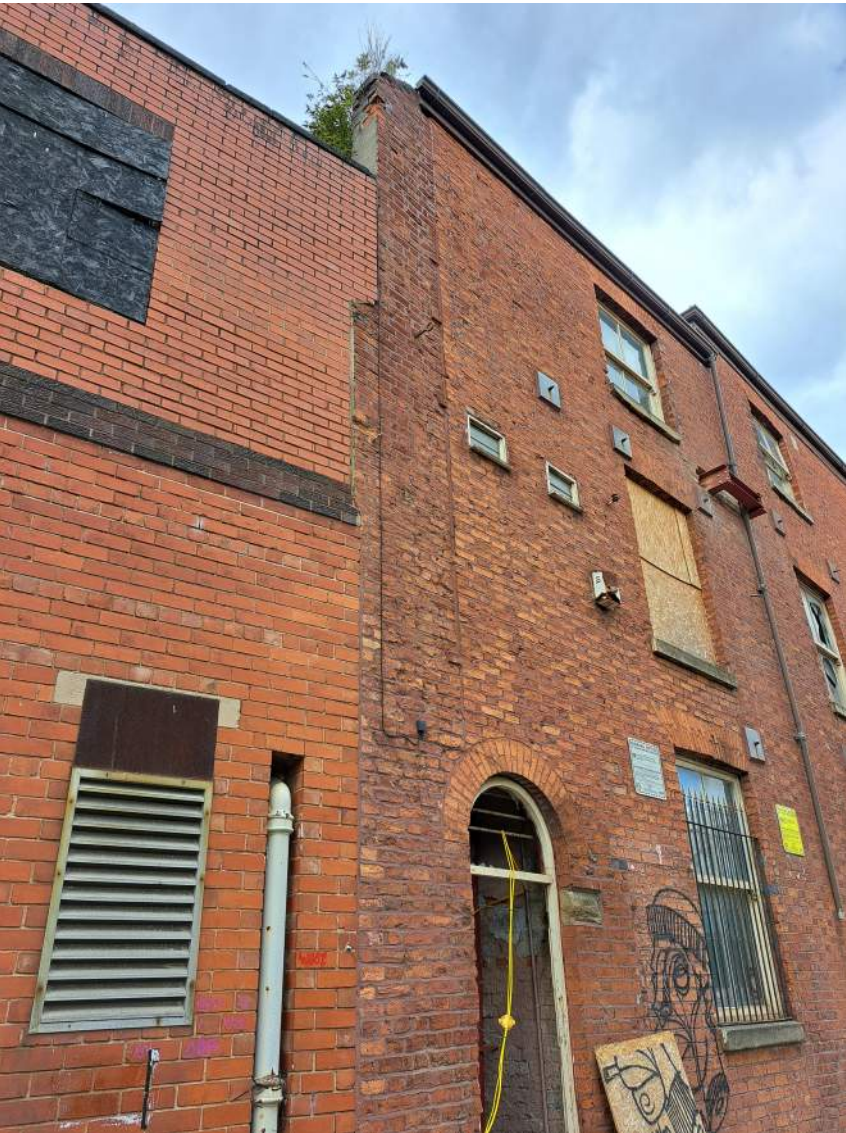
E08: JOINT BETWEEN 19TH AND 20TH CENTURY SECTIONS OF 123 LIVERPOOL ROAD ON OLD MEDLOCK STREET. VEGETATION GROWTH IS VISIBLE AT ROOF LEVEL.
