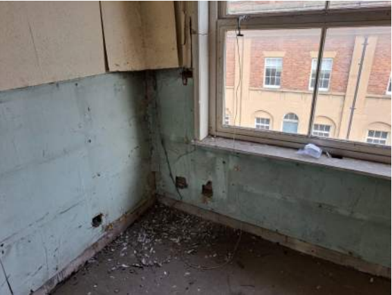
218: CRACKING OF FINISHES PROPAGATING FROM CORNER OF WINDOW OPENING ON LIVERPOOL ROAD ELEVATION IN ROOM 208.
