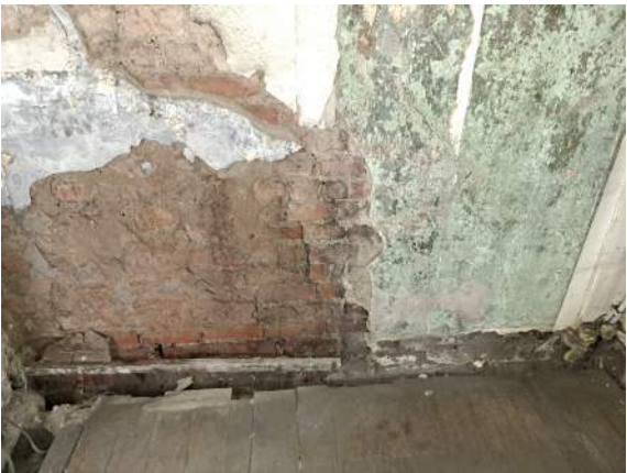
204: MINOR CRACKING OF EXTERNAL WALL OF WOOLLAM PLACE IN ROOM 202.
