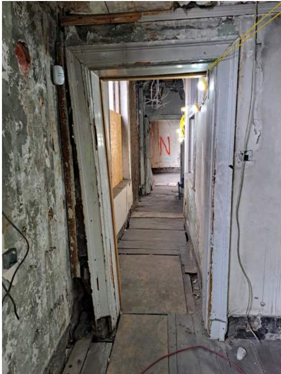
111: VISIBLE DISTORTION OF DOOR FRAME BETWEEN ROOMS 104 AND 109 IN RELATION TO ADJACENT EXTERNAL WALL ON WOOLLAM PLACE WHICH SHOWS SIGNS OF MOVEMENT.
