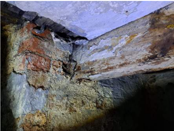
B02: THE ENDS OF THE TIMBER BEAMS OVER ROOM B02 WHERE THEY ARE EMBEDDED INTO THE EXTERNAL WALL ON LIVERPOOL ROAD SHOW SIGNS OF DECAY.
