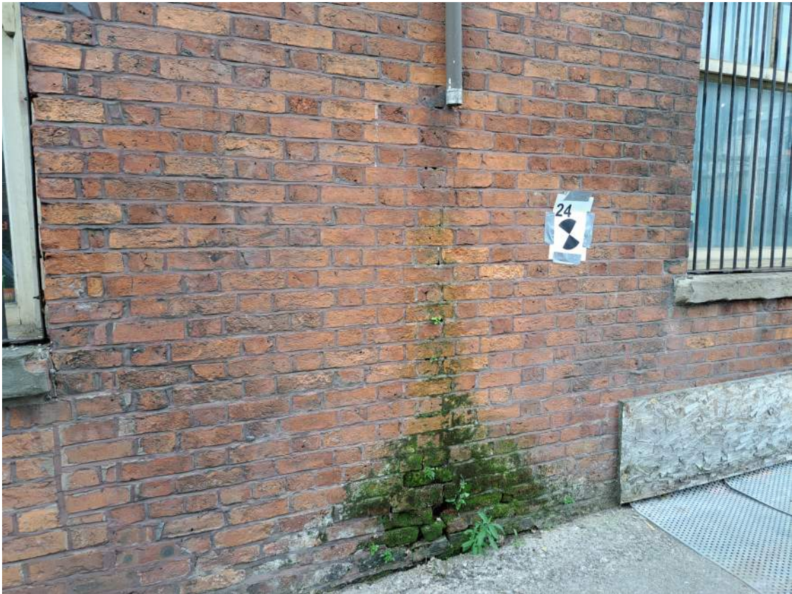
E07: WEATHERED MORTAR JOINTS, SATURATED BRICKWORK AND VEGETATION GROWTH UNDER A RAINWATER DOWNPIPE ON THE EAST ELEVATION TO 123 LIVERPOOL ROAD.
