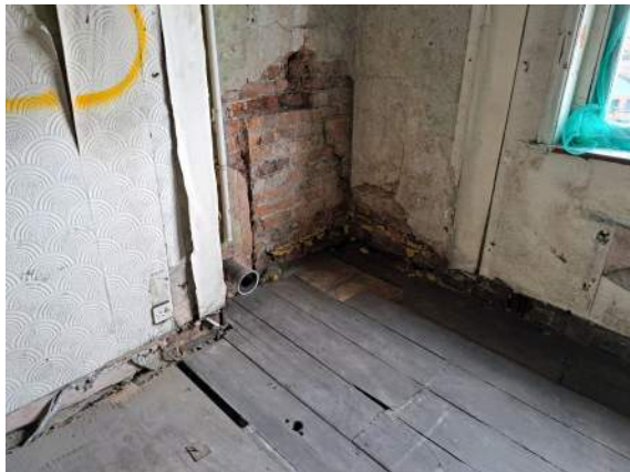
211: CRACKING OF MASONRY ON REAR ELEVATION OF ROOM 206.
