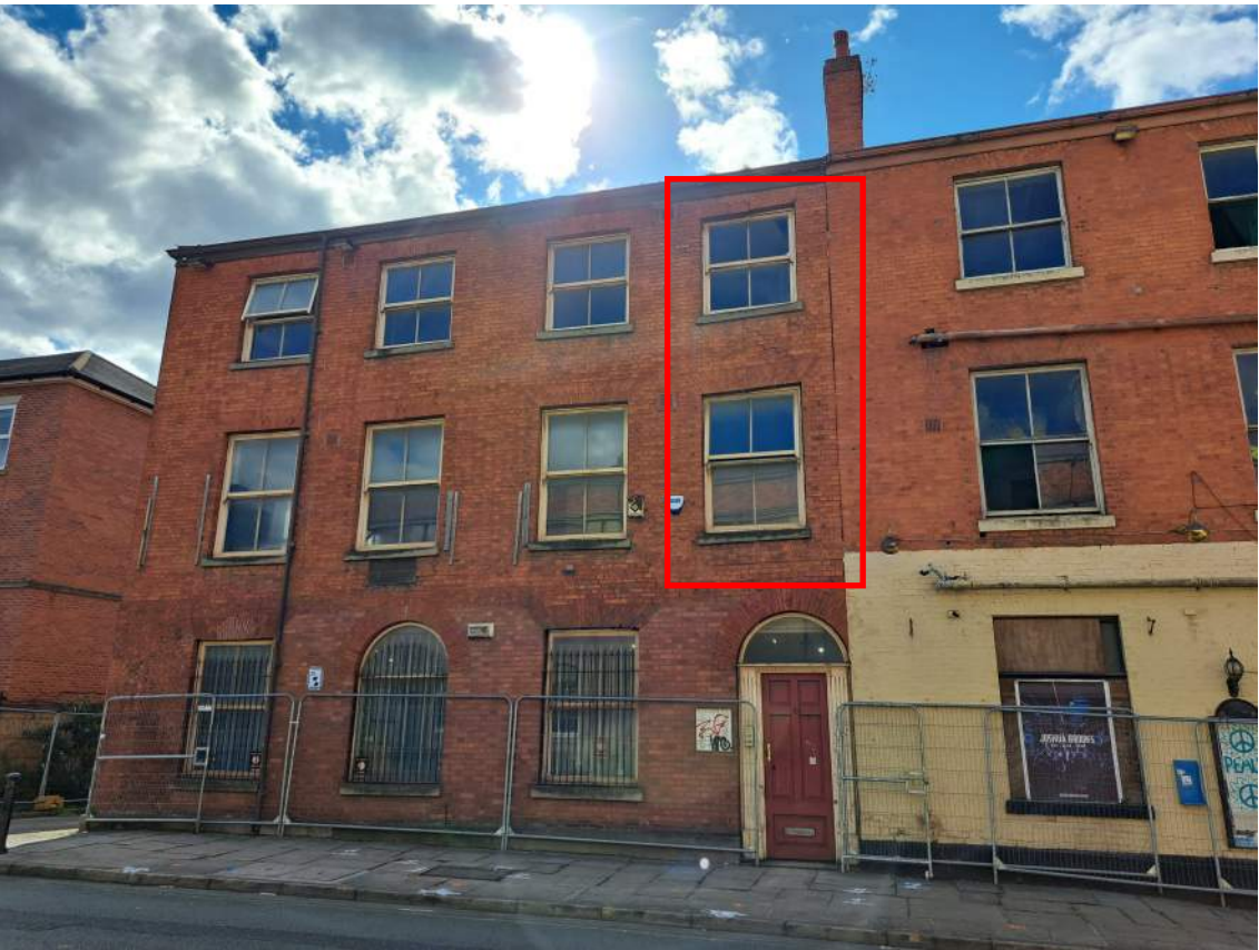
E10: GENERAL VIEW OF NORTH ELEVATION TO 123 LIVERPOOL ROAD. BRICKWORK APPEARS TO BE IN SOUND CONDITION GENERALLY. THERE ARE SOME SIGNS OF HISTORIC MOVEMENT, PARTICULARLY IN THE AREA INDICATED.
