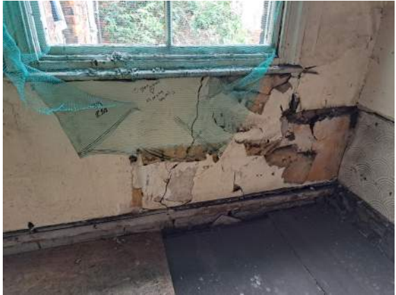
207: VERTICAL CRACK UNDER WINDOW OPENING ON THE EAST ELEVATION OF ROOM 204.
