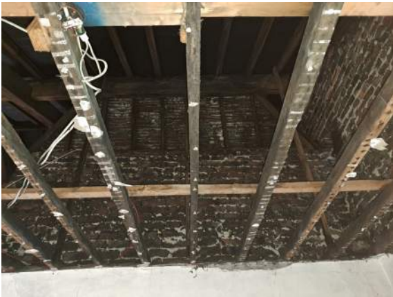
205: MASONRY/STUDWORK ENCLOSURE FORMING SKYLIGHT ABOVE THE STAIRWELL VIEWED FROM ROOM 201. SIGNS OF DAMP ON SURFACE OF TIMBER ROOF PURLIN ADJACENT TO ENCLOSURE.
