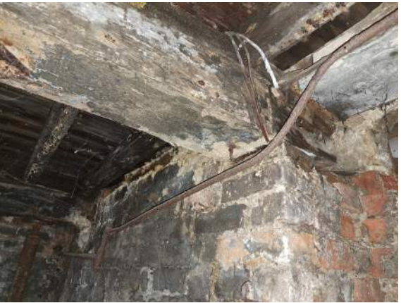
B24: EVIDENCE OF DECAY AT THE BEARING OF A TIMBER BEAM OVER ROOM B11 WHERE IT IS EMBEDDED INTO THE EXTERNAL WALL ON LIVERPOOL ROAD.
