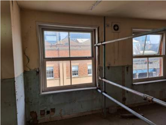
216: MINOR CRACKING AROUND WINDOW OPENING IN EXTERNAL WALL ON LIVERPOOL ROAD AS VIEWED FROM WITHIN ROOM 208.
