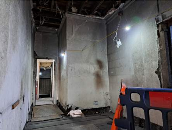
104: SECTION OF MASONRY MISSING AT BOTTOM CORNER OF LOAD-BEARING WALL WITHIN ROOM 104.
