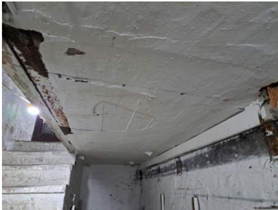
B01: FILLER JOIST FLOOR AT GROUND FLOOR OVER ROOM B01. THERE ARE SIGNS OF CORROSION ON THE UNDERSIDE OF THE STEEL JOISTS.
