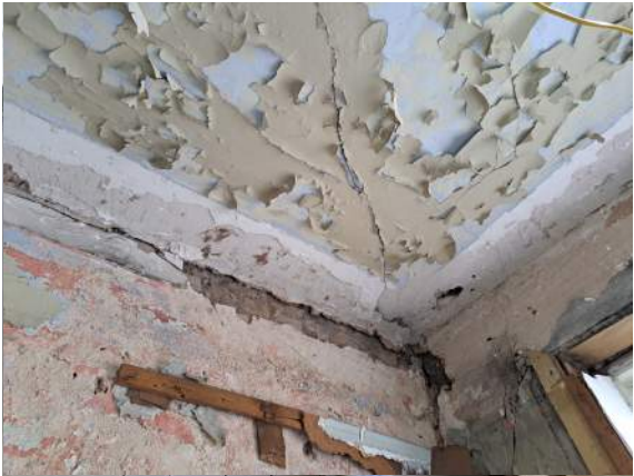
117: EXTENSIVE CRACKING OF CEILING FINISHES OVER ROOM 107. A GAP ALSO APPEARS TO HAVE OPENED UP BETWEEN THE CEILING AND THE INTERNAL WALL SEPARATING 123 AND 125 LIVERPOOL ROAD.
