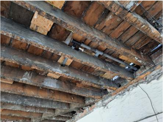
102: VARIOUS NOTCHES HAVE BEEN FORMED THROUGH TIMBER FLOOR JOISTS AT 2ND FLOOR OVER ROOM 103.
