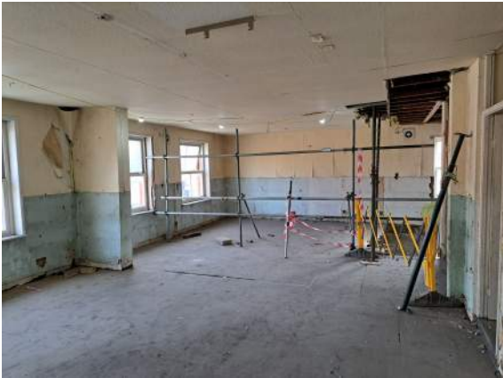
215: GENERAL VIEW OF ROOM 208. SECTION OF 2ND FLOOR IS INACCESSIBLE ON OLD MEDLOCK STREET SIDE OF BUILDING DUE TO COLLAPSE.
