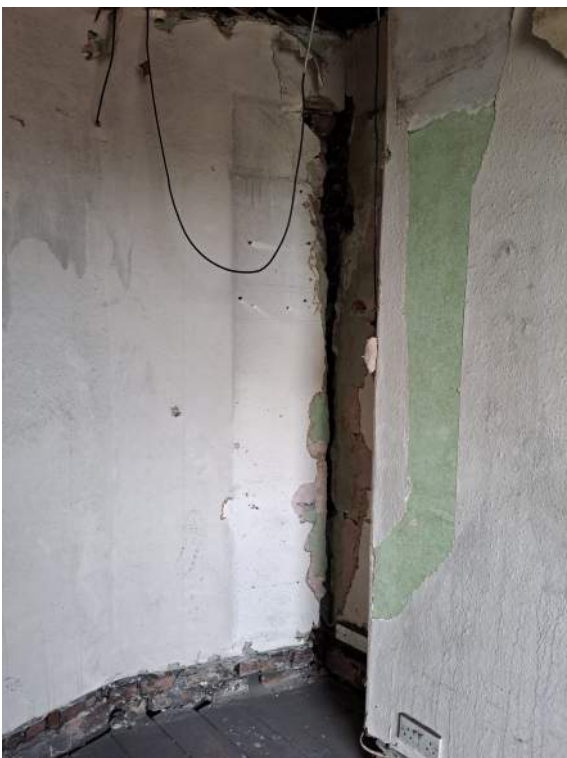
213: 100mm GAP BETWEEN WALLS IN SOUTH EAST CORNER OF ROOM 205. THERE IS ALSO AN OBVIOUS DIP IN THE TIMBER FLOOR OF THIS ROOM TOWARDS THE NORTH EAST CORNER.
