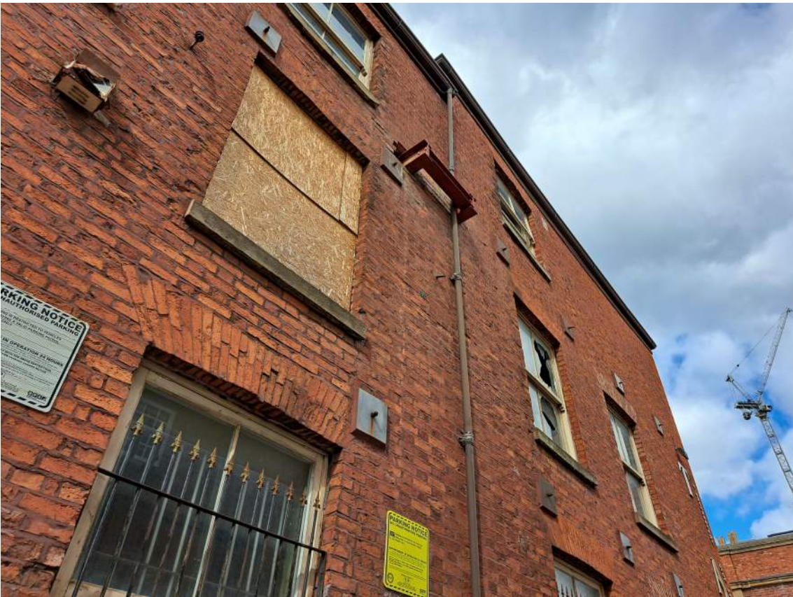
E05: EAST ELEVATION TO 123 LIVERPOOL ROAD. THERE IS A VISIBLE BOW TO THE GABLE WALL AS WELL AS SEVERAL PATTRESS PLATES BUT THERE ARE NO OBVIOUS SIGNS OF ONGOING MOVEMENT.
