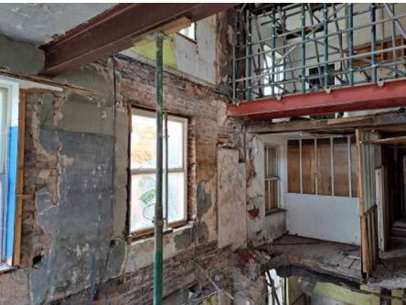
114: MASONRY ON INTERNAL FACE OF EXTERNAL WALL IS IN VARIABLE CONDITION ADJACENT TO COLLAPSE ZONE WITHIN REAR SECTION OF 123 LIVERPOOL ROAD. EVIDENCE THAT TIE RODS HAVE ALSO FAILED WHEN FLOOR HAS COLLAPSED.
