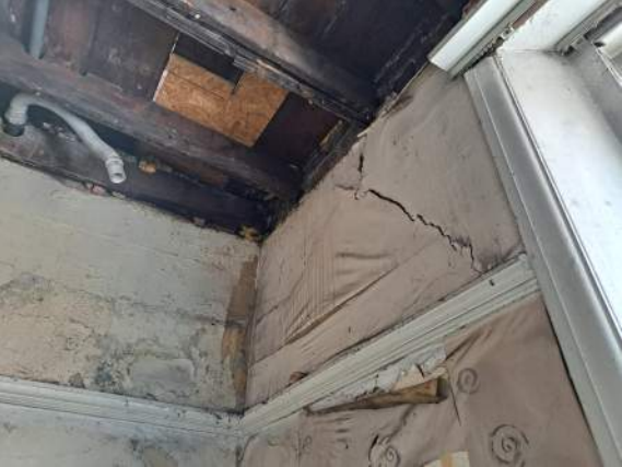
110: CRACKING OF FINISHES ON INTERNAL FACE OF EXTERNAL WALL ON WOOLLAM PLACE IN ROOM 105.
