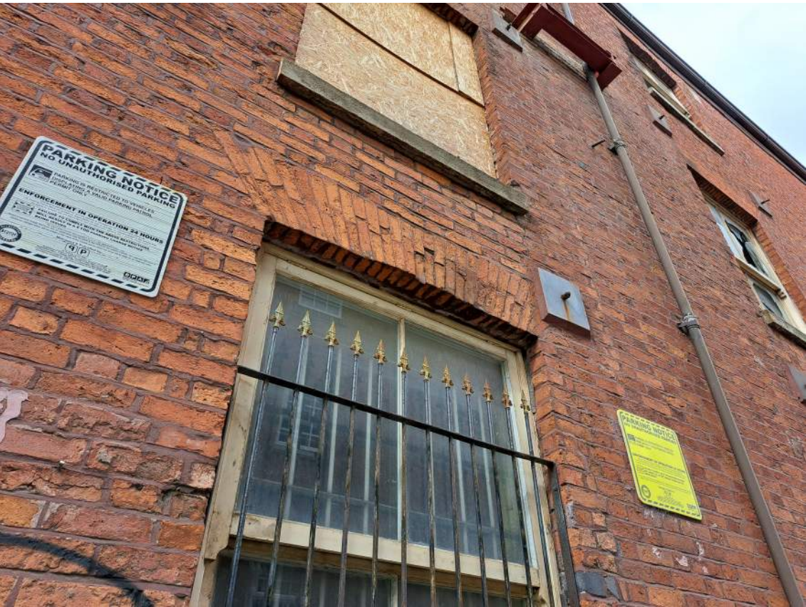
E06: DISPLACED BRICKS IN A FLAT ARCH ABOVE A WINDOW OPENING ON THE EAST ELEVATION TO 123 LIVERPOOL ROAD.
