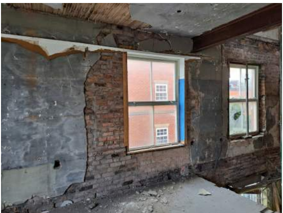
113: CRACKING OF MASONRY OVER WINDOW OPENING WITHIN INACCESSIBLE AREA OF ROOM 107 ON OLD MEDLOCK STREET ELEVATION.
