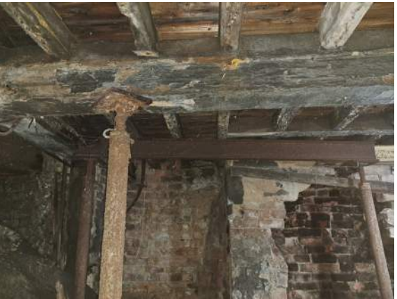
B23: HISTORIC PROPPING TO TIMBER BEAMS SUPPORTING THE GROUND FLOOR OVER ROOM B11. AS WITH ROOM B10, THE BEAMS AND JOISTS IN THIS AREA APPEAR TO BE IN VARIABLE CONDITION.
