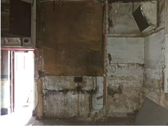
G07: CRACKING OF FINISHES ON INTERNAL FACE OF REAR EXTERNAL WALL TO ROOM G03. IT IS NOT CLEAR WHETHER THE CRACKING IS REFLECTED IN THE MASONRY BEHIND.
