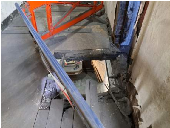
103: APPARENT FIRE DAMAGE OF TIMBER JOISTS AROUND OPENING THROUGH FLOOR IN ROOM 104. ACCESS INTO ADJACENT BATHROOM IS NOT POSSIBLE DUE TO UNSAFE STRUCTURE.
