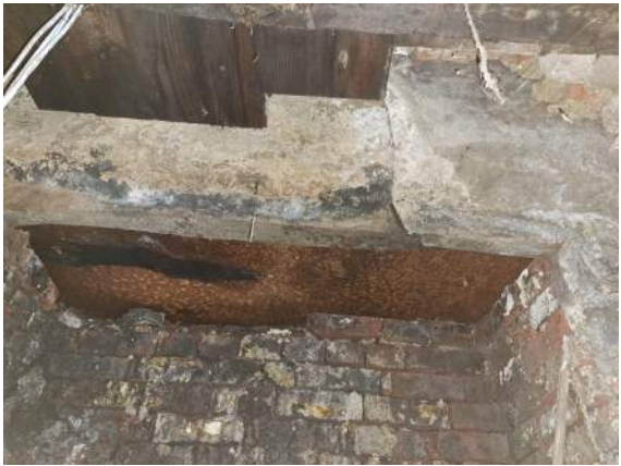
B27: CRACK IN STONE LINTEL ABOVE INFILLED PAVEMENT LIGHT ON THE LIVERPOOL ROAD ELEVATION OF ROOM B13.
