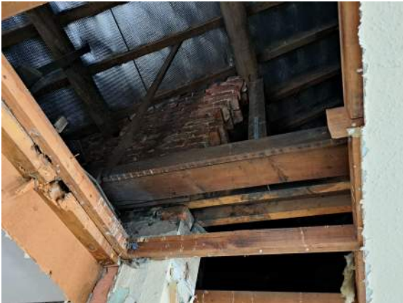
219: TIMBER BEAM AND POST SUPPORTING ROOF PURLINS IS VISIBLE FROM OPENING IN CEILING OVER ROOM 208. THIS APPEARS TO BE HAVE BEEN INSTALLED TO ALLOW FOR THE REMOVAL OF A LOAD-BEARING WALL WHICH WOULD HAVE HISTORICALLY SUB-DIVIDED THE ROOM.
