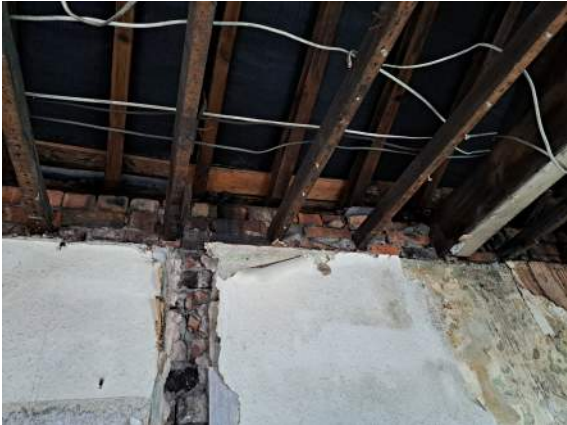
208: SIGNS OF DAMP AND WATER INGRESS THROUGH THE TIMBER WALL PLATE AT EAVES LEVEL OF ROOM 206.
