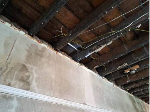
109: VARIOUS NOTCHES HAVE BEEN FORMED THROUGH END OF TIMBER FLOOR JOISTS OVER ROOM 105.
