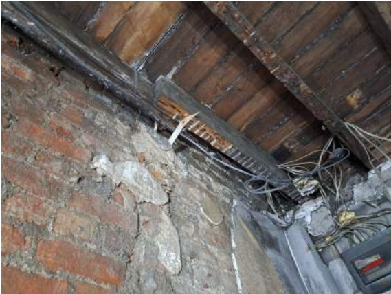
105: SPLICED SECTION OF TIMBER JOISTS ADJACENT TO EXTERNAL WALL ON WOOLLAM PLACE IN ROOM 104.
