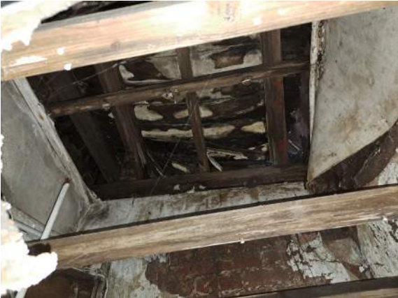
G10: FAILED TIMBER FLOOR OVER REAR SECTION OF CORRIDOR IN ROOM G06. SIGNIFICANT WATER INGRESS IS APPARENT IN THIS PART OF THE STRUCTURE.
