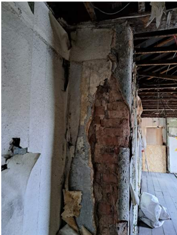
214: VERTICAL CRACK IN MASONRY ADJACENT TO DOOR OPENING INTO ROOM 206 AS SEEN FROM ROOM 202.
