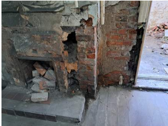
G06: SECTION OF MASONRY CHIMNEY BREAST HAS COLLAPSED ON REAR ELEVATION OF ROOM G02.
