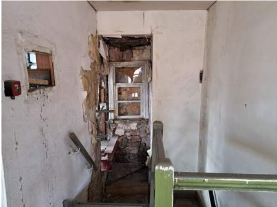
220: SECTION OF EXTERNAL WALL TO THE REAR OF THE INACCESSIBLE STAIR CORE ADJACENT TO ROOM 208 IS IN POOR CONDITION.
