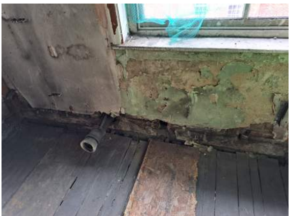
212: GAP BETWEEN TIMBER FLOOR AND EXTERNAL WALL ON WOOLLAM PLACE IN ROOM 205.
