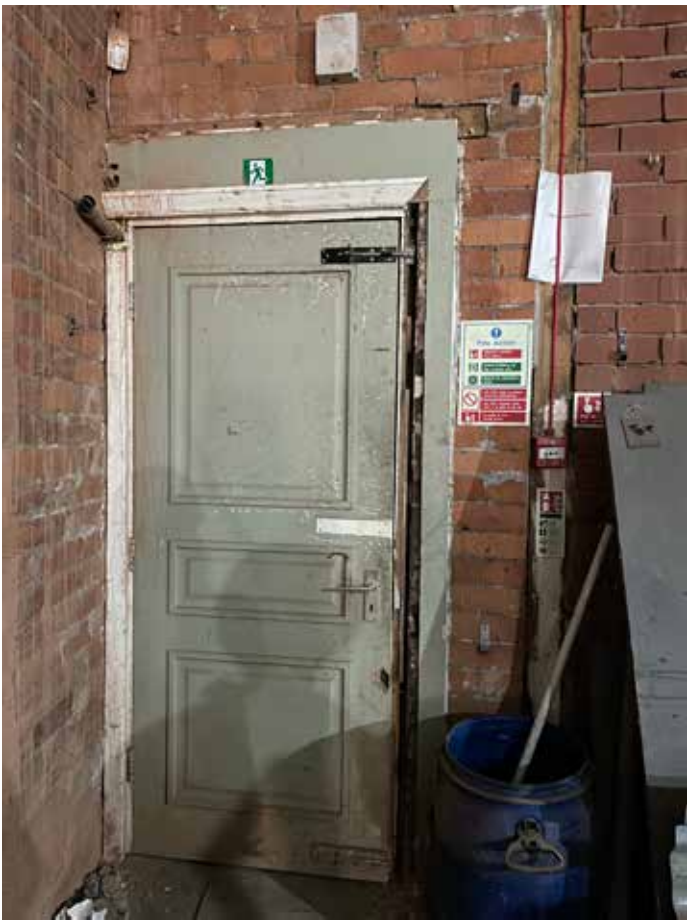
Image: Loading bay door requiring minor enlargement.
