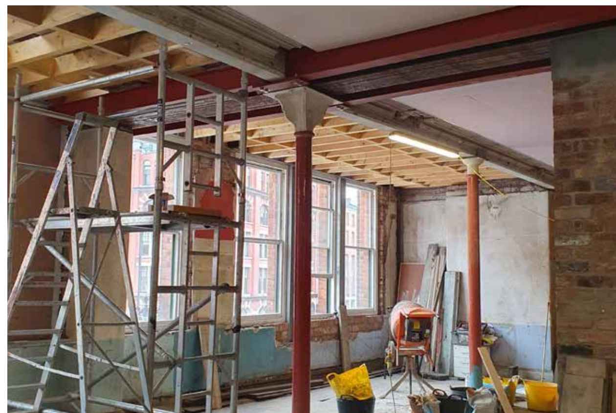
Images: (Above) unsupported chimney breast and (below) additional stabilising works.
