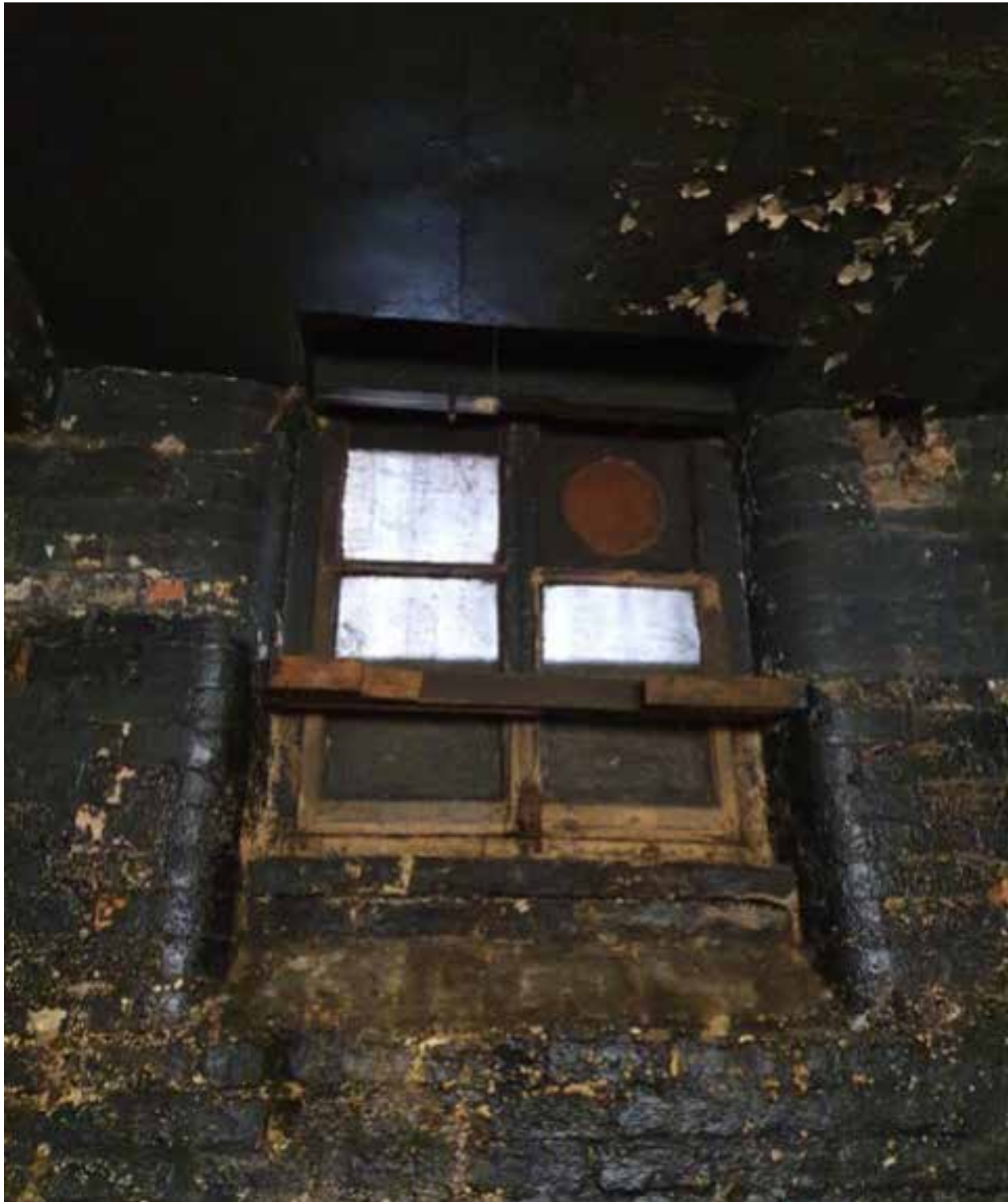
Image: Non-original alterations to basement windows to Back Piccadilly.
