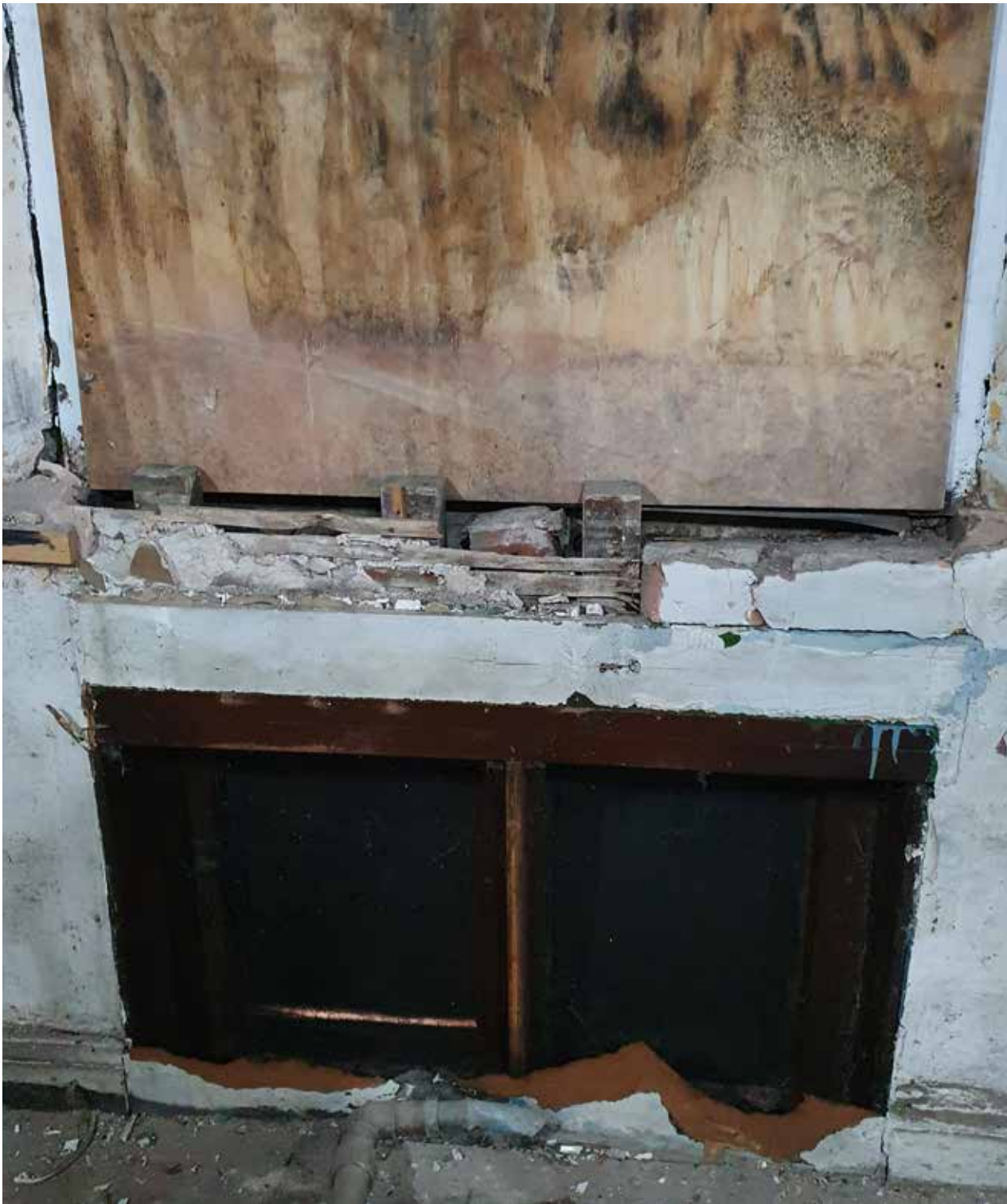
Image: Non-original alterations to windows to Back Piccadilly where floor is bi-secting windows.
