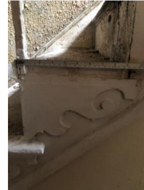
3. Replace missing nosings
