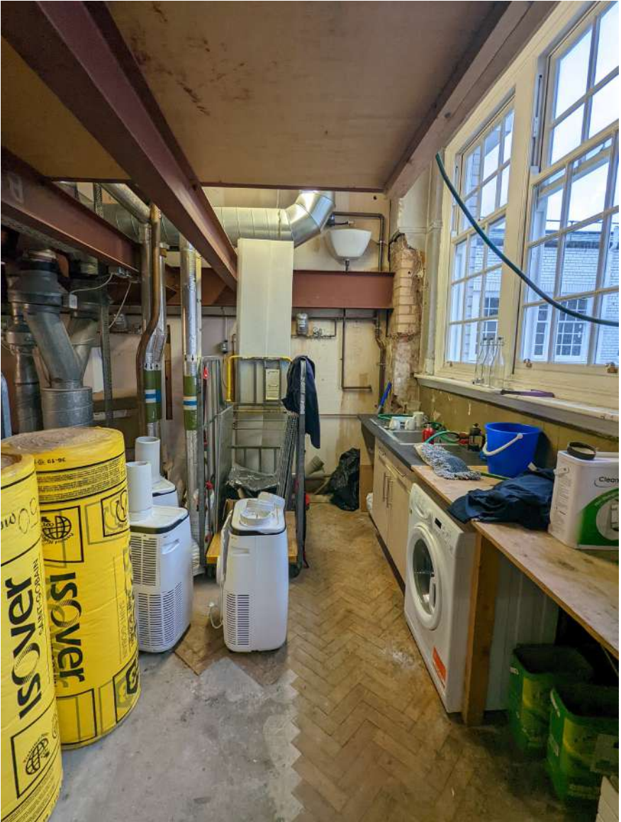
Unkempt maintenance and plant equipment to be removed.
