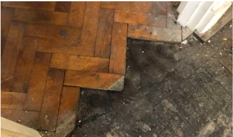
B. INFILL TO PARQUETE FLOORING IN PLACES
