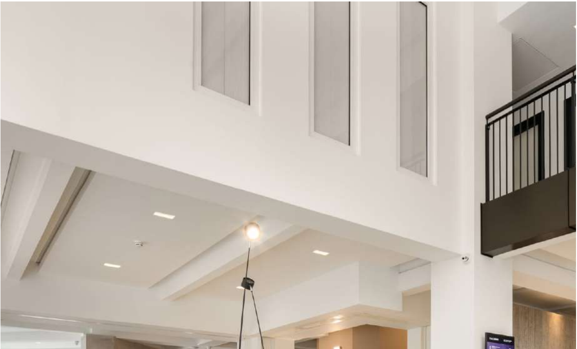
EXISTING RECESSED DOWNLIGHTS
