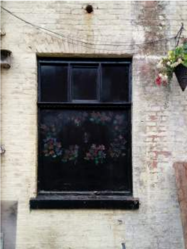
S05. No. 125 windows to be restored.
