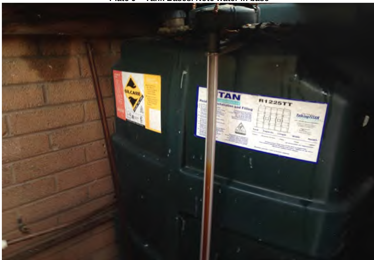
Plate 10 – Oil Tank in Southeastern Corner of Property
