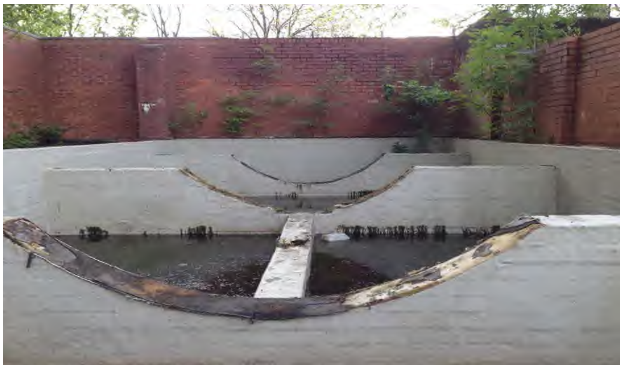
Plate 9 – Tank Bases. Note water in base
