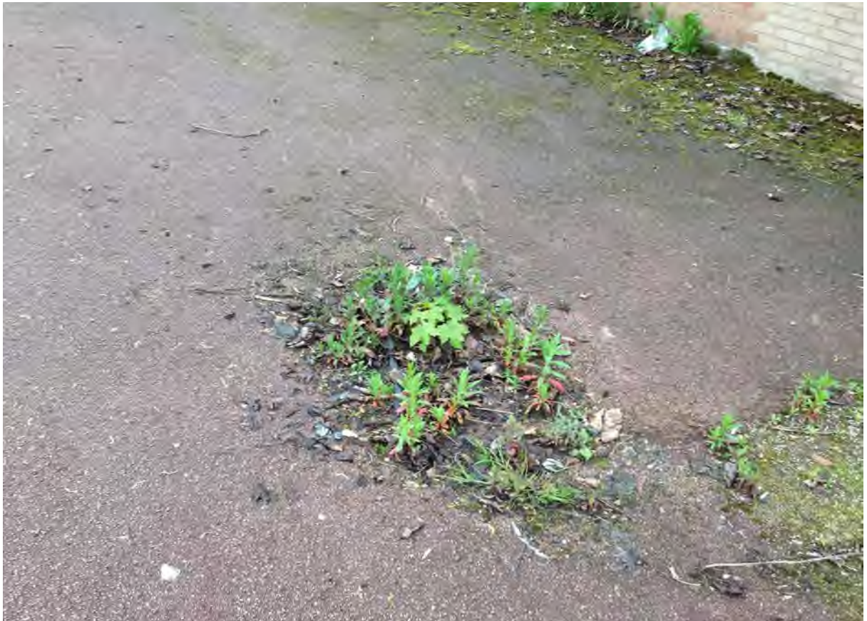
Plate 15 - Area of surface settlement in Northern Car Park
