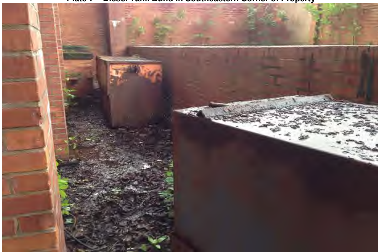
Plate 8 – Diesel Tank Bund in Southeastern Corner of Property
