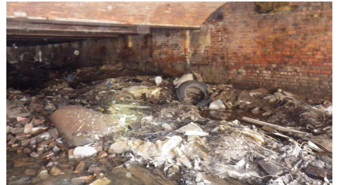
Figure 5-3 Debris build up within culvert
