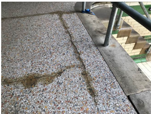
Cracks in terrazzo finished filler joist floors around the edge of the Females Pool
