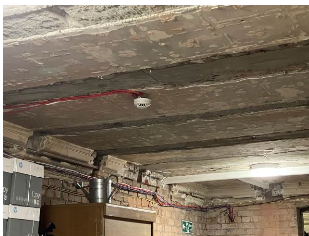
Plastic clips to poorly fixed cabling in the basement
