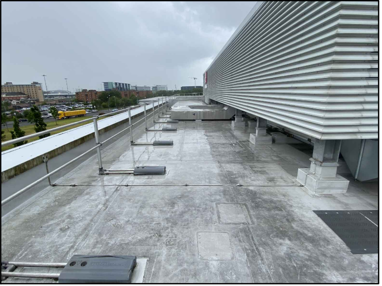
Area F Approximate area 25m 2 No. of PV panels 5 Output = 2.76kW p
