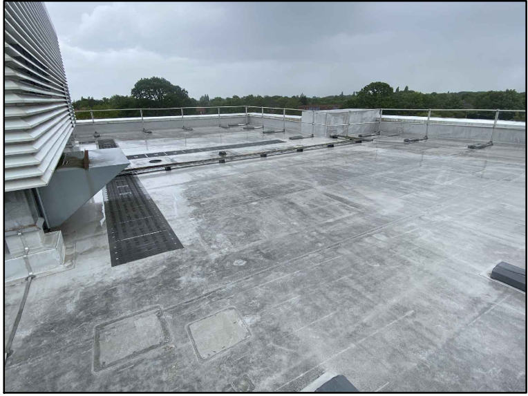
Area E Approximate area 90m 2 No. of PV panels 30 Output = 13.8kW p
