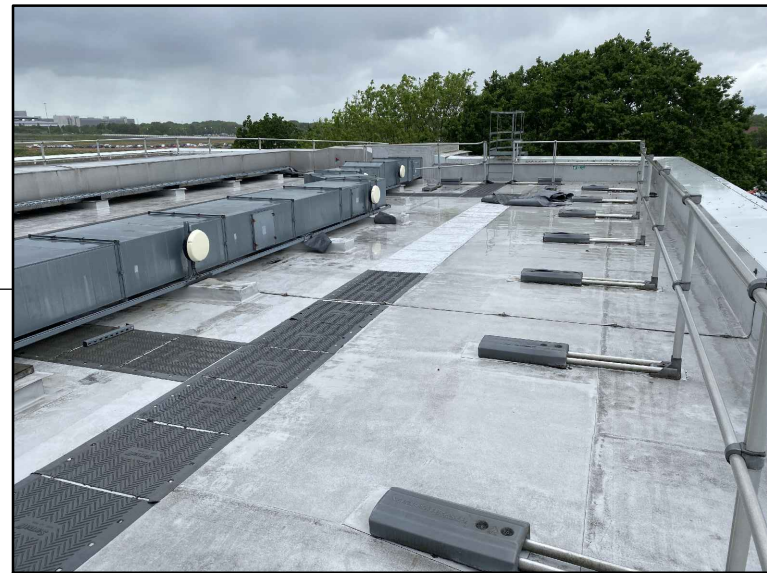
Area C Approximate area 40m 2 No. of PV panels 12 Output = 5.52kW p
