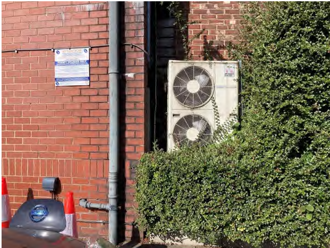
Plate 5 – AC units present adjacent to site entrance.
