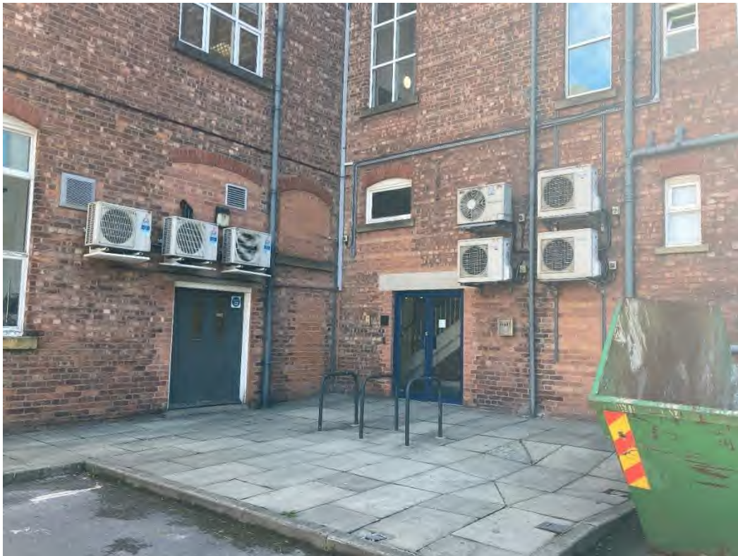
Plate 7 – AC units present in southwest corner of Greenheys building, looking northeast.
