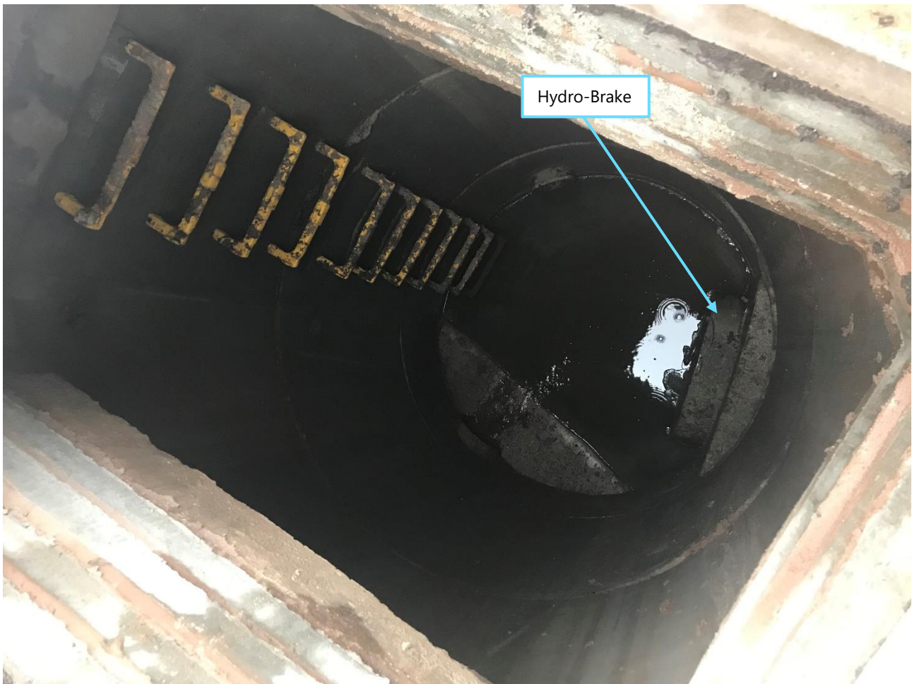
Figure 2-9 Hydro-Brake installed in MHSW-00-02
