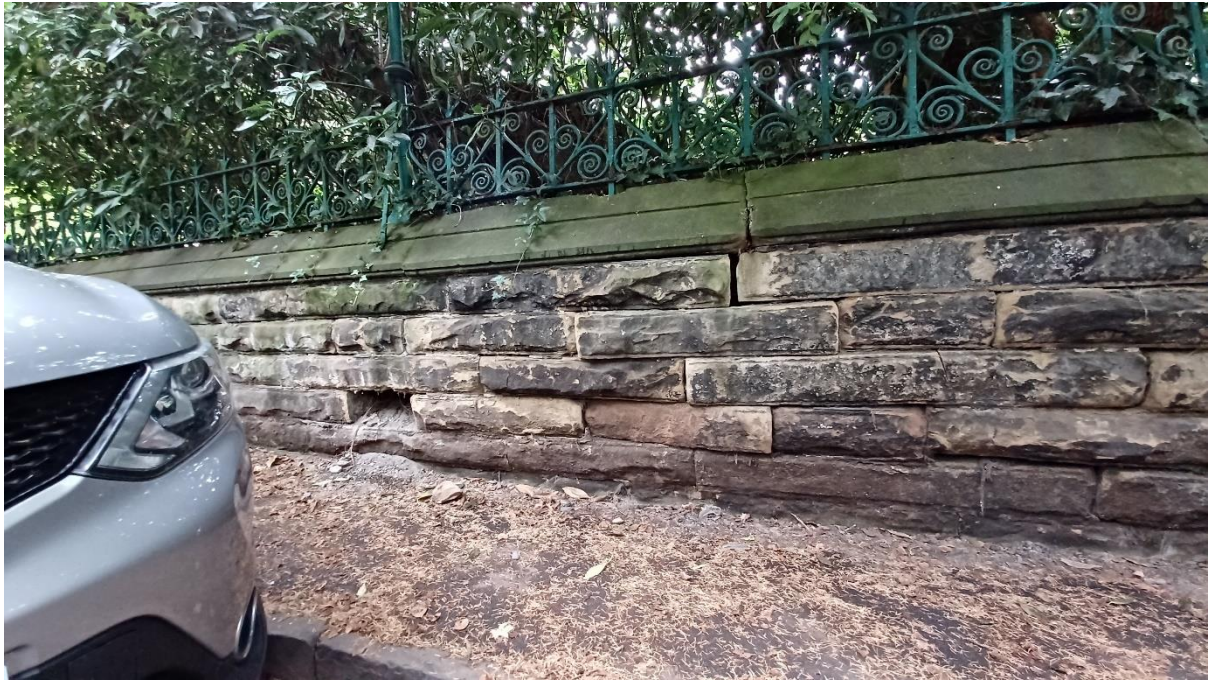
Photo 5: Boundary wall with missing stone and visible movement of stones, Photo taken in August 2022.
