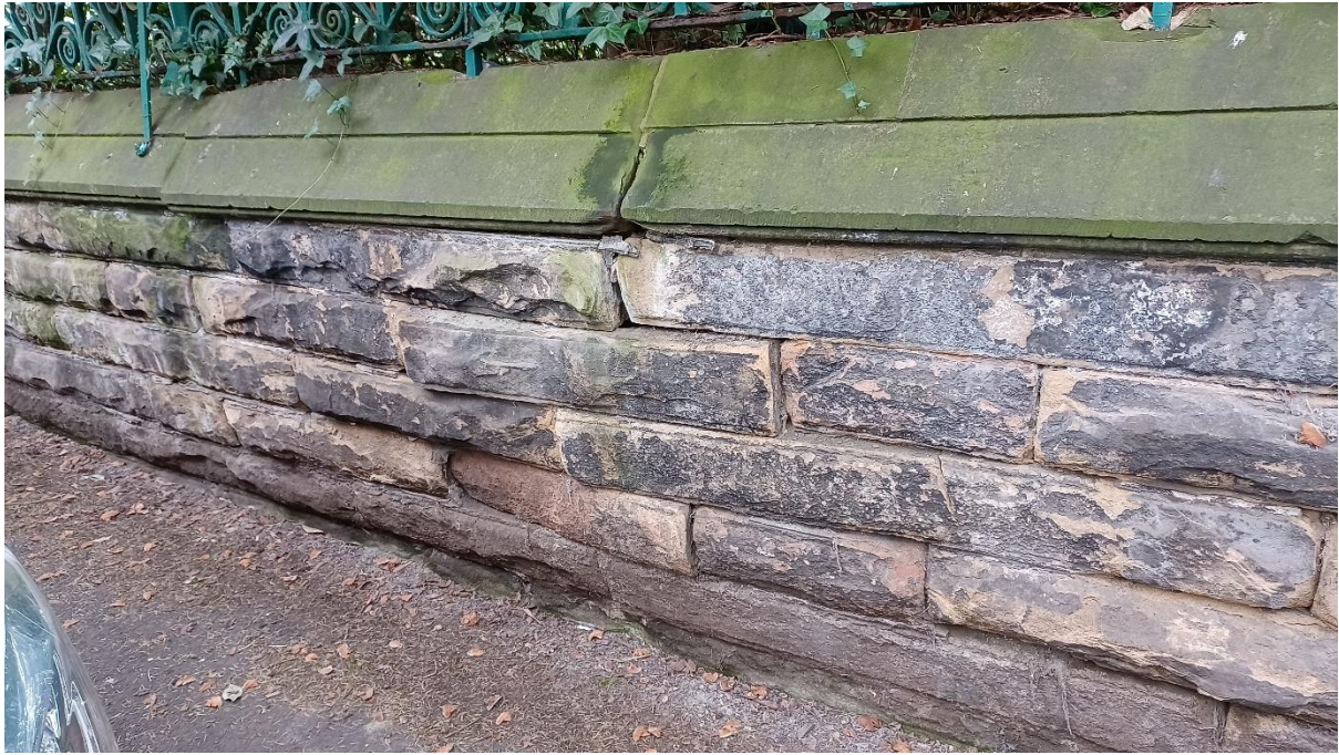
Photo 1: St James Church boundary/retaining wall on Stenner Lane, visible cracking and bulging of wall
