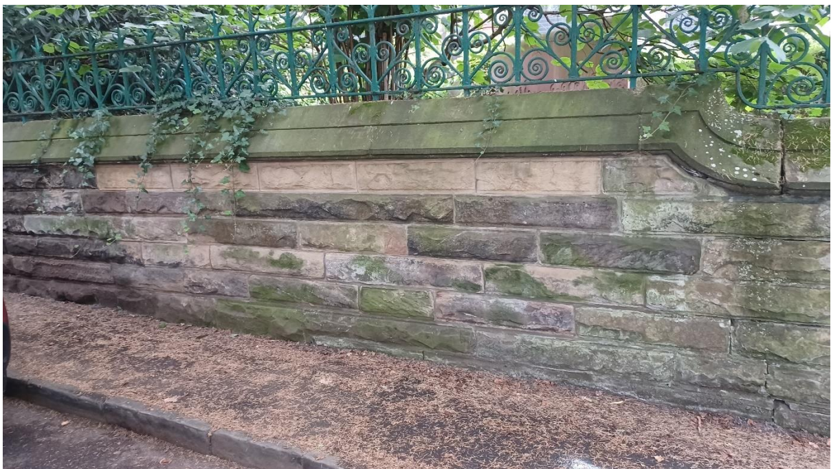
Photo 6: Boundary wall showing areas of previous wall repairs and stone replacement on Stenner Lane.
