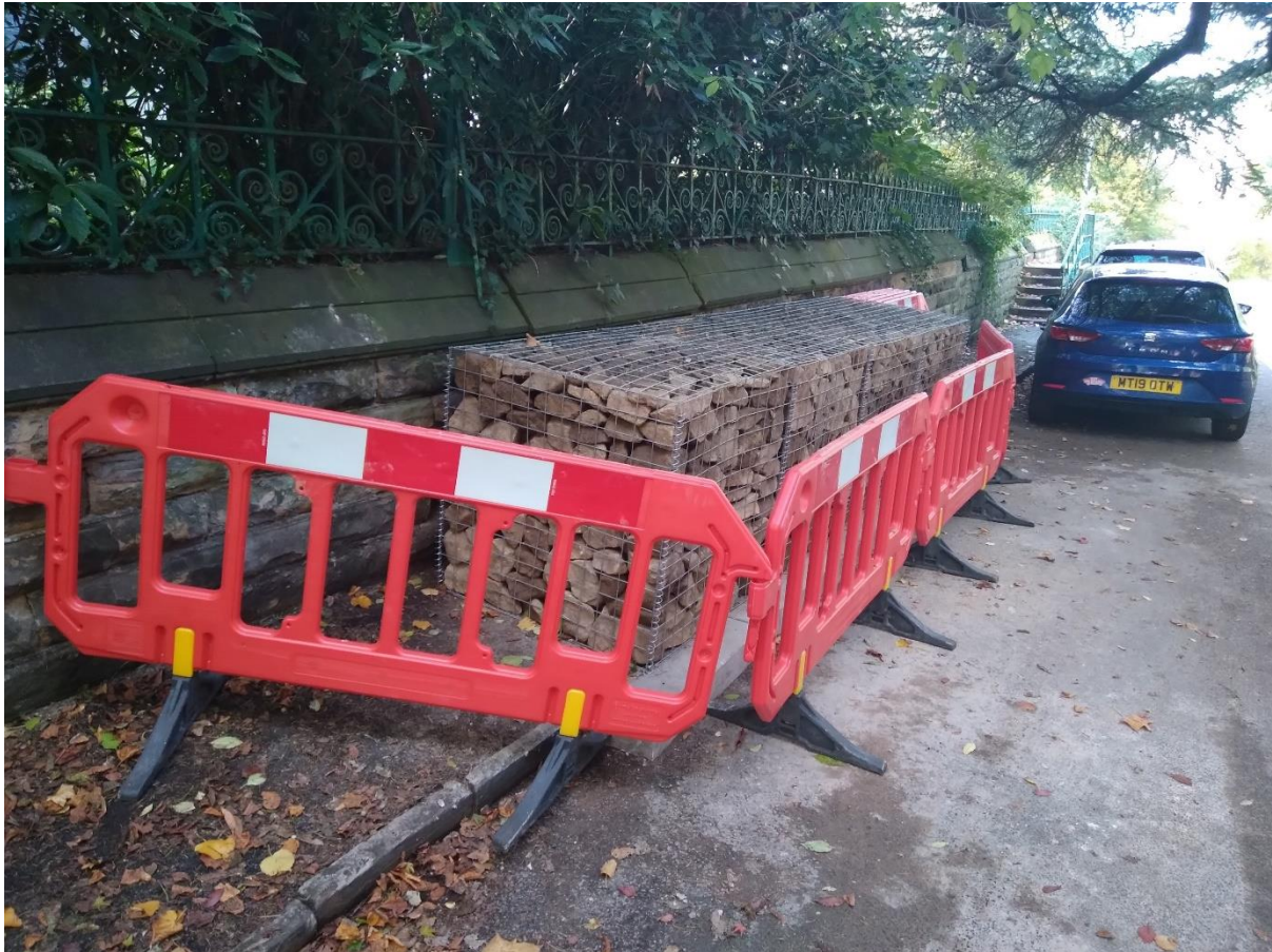
Photo 9: Gabion baskets with temporary fencing around. Photograph taken in October 2022.
