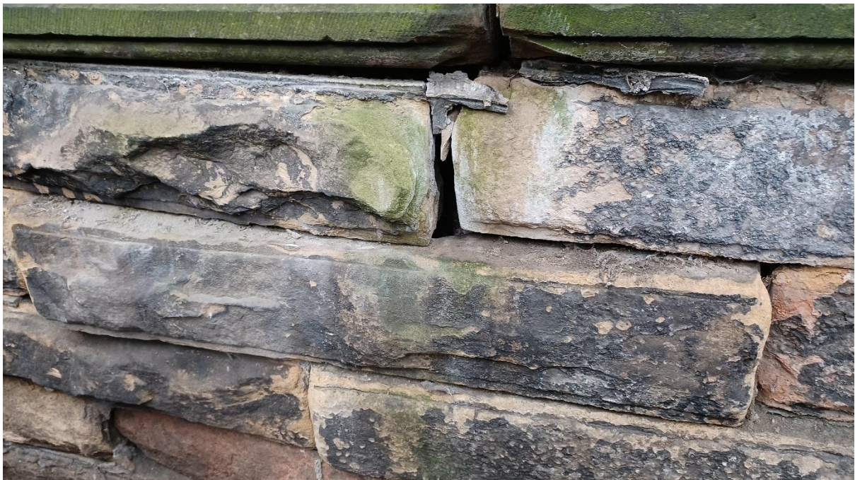
Photo 2: Holes and missing mortar formed in retaining wall between stone wall sections caused by movement.
