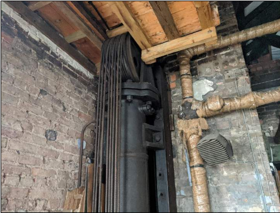
Plate 73: lift/hoist mechanism adjacent to goods lift
