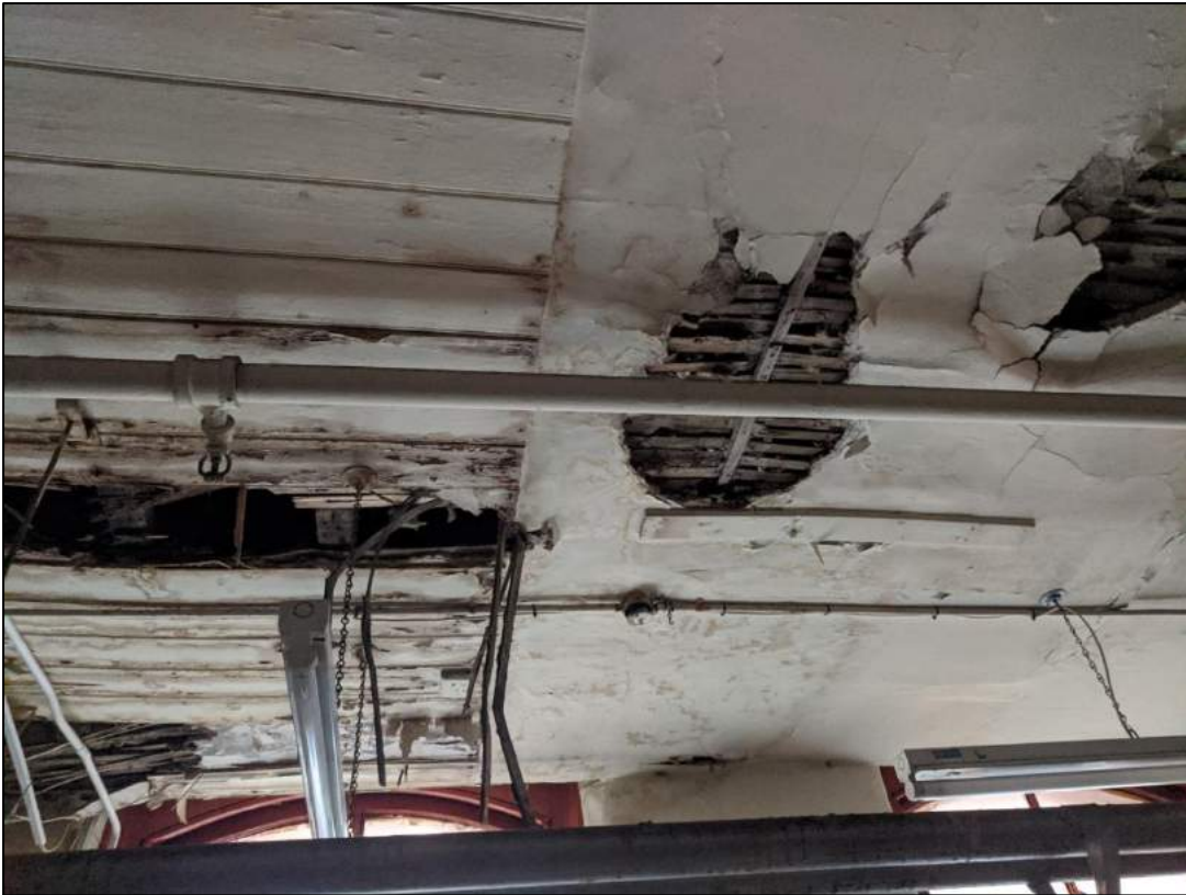
Plate 35: Decayed timber and lath and plaster ceiling
