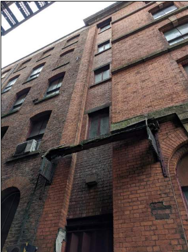
Plate 16: Recessed loading bay and straight joint (to left)
