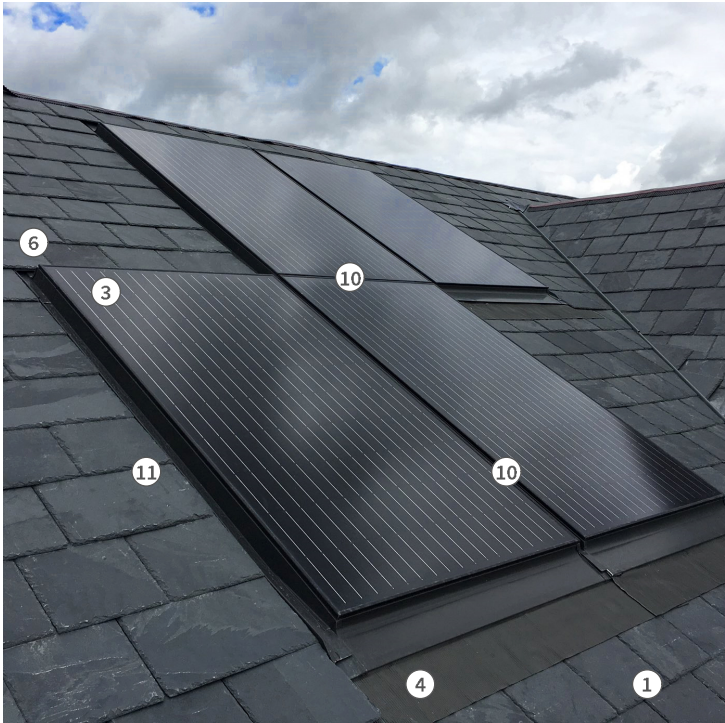
Image 02 [NTS] Completed installation of integrated photovoltaic panels
