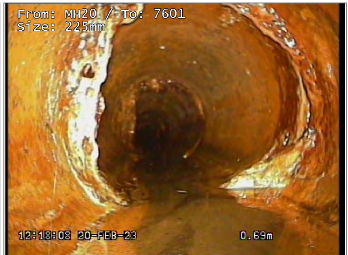
Attached deposits, encrustation from 7 to 4 o'clock 15% cross-sectional area loss
