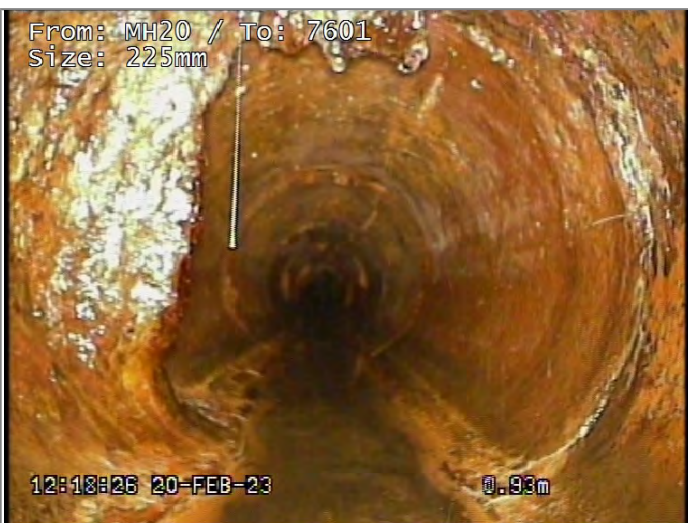
Attached deposits, encrustation from 8 to 12 o'clock 25% cross-sectional area loss
