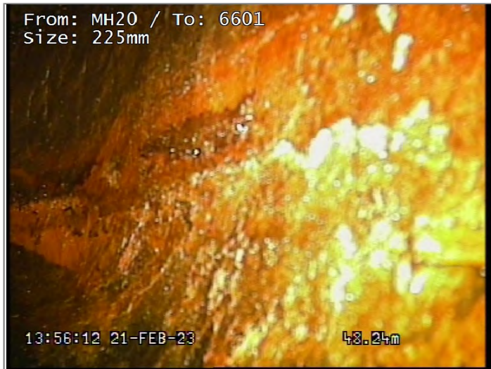
Finish node type, manhole, reference 6601
