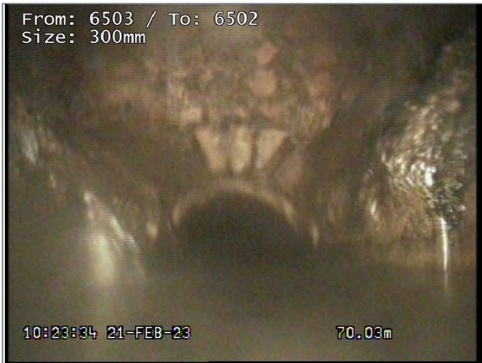
Finish node type, manhole, reference 6502
