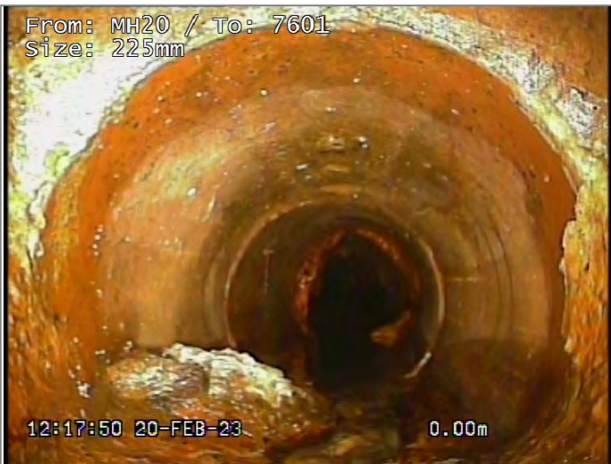
Settled deposits hard or compacted 25% cross-sectional area loss
