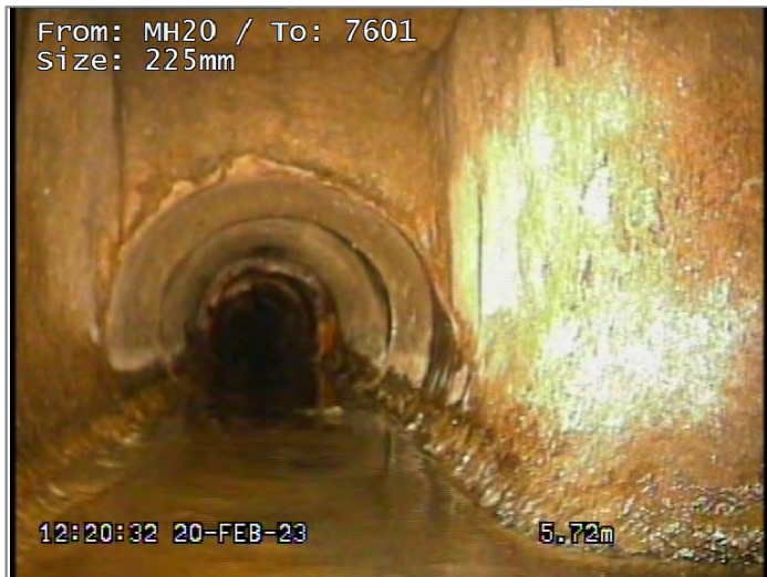
Finish node type, manhole, reference 7601
