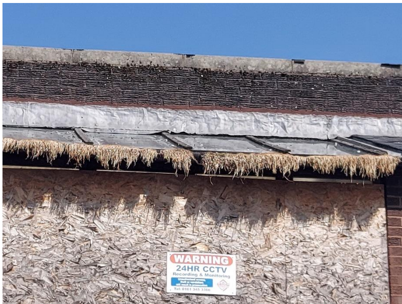
PLATE 4 SHOWING LIFTED LEAD FLASHING
