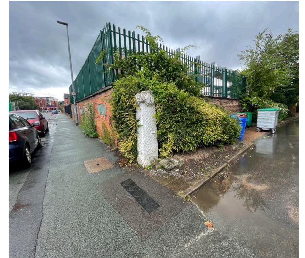
FIGURE 14: POOLING AND OVERGROWN BUSHES
