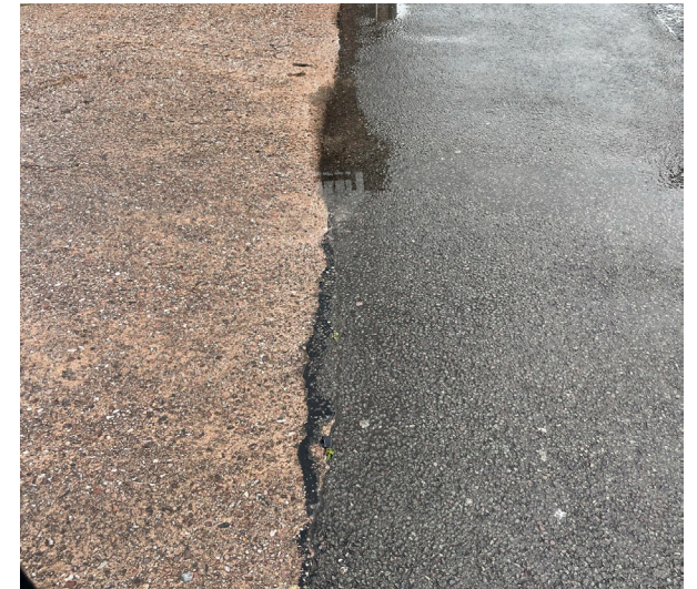
FIGURE 5: POOLING BETWEEN ENTRANCE AND HIGHWAY
