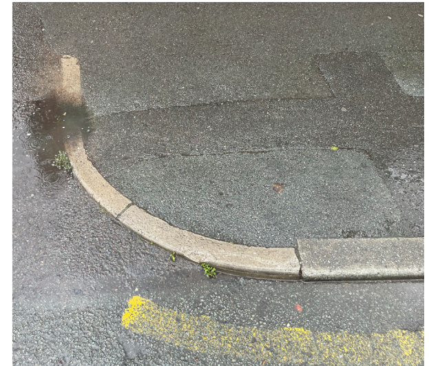
FIGURE 9: FADED YELLOW LINES
