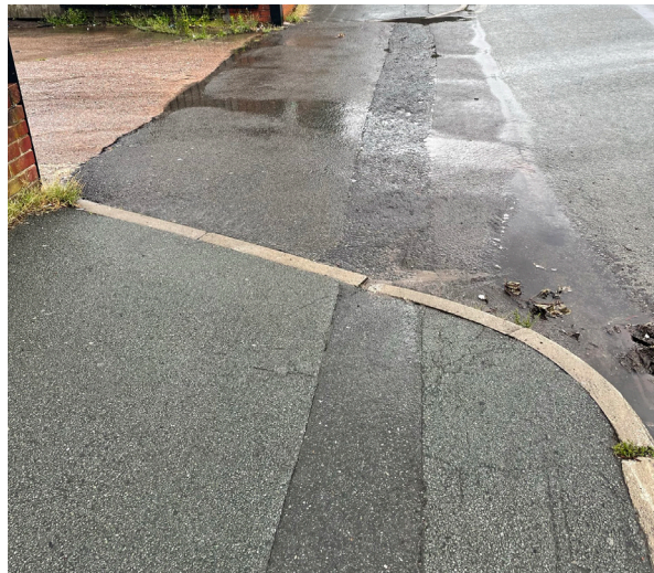
FIGURE 6: BLOCKED DRAIN & PONDING
