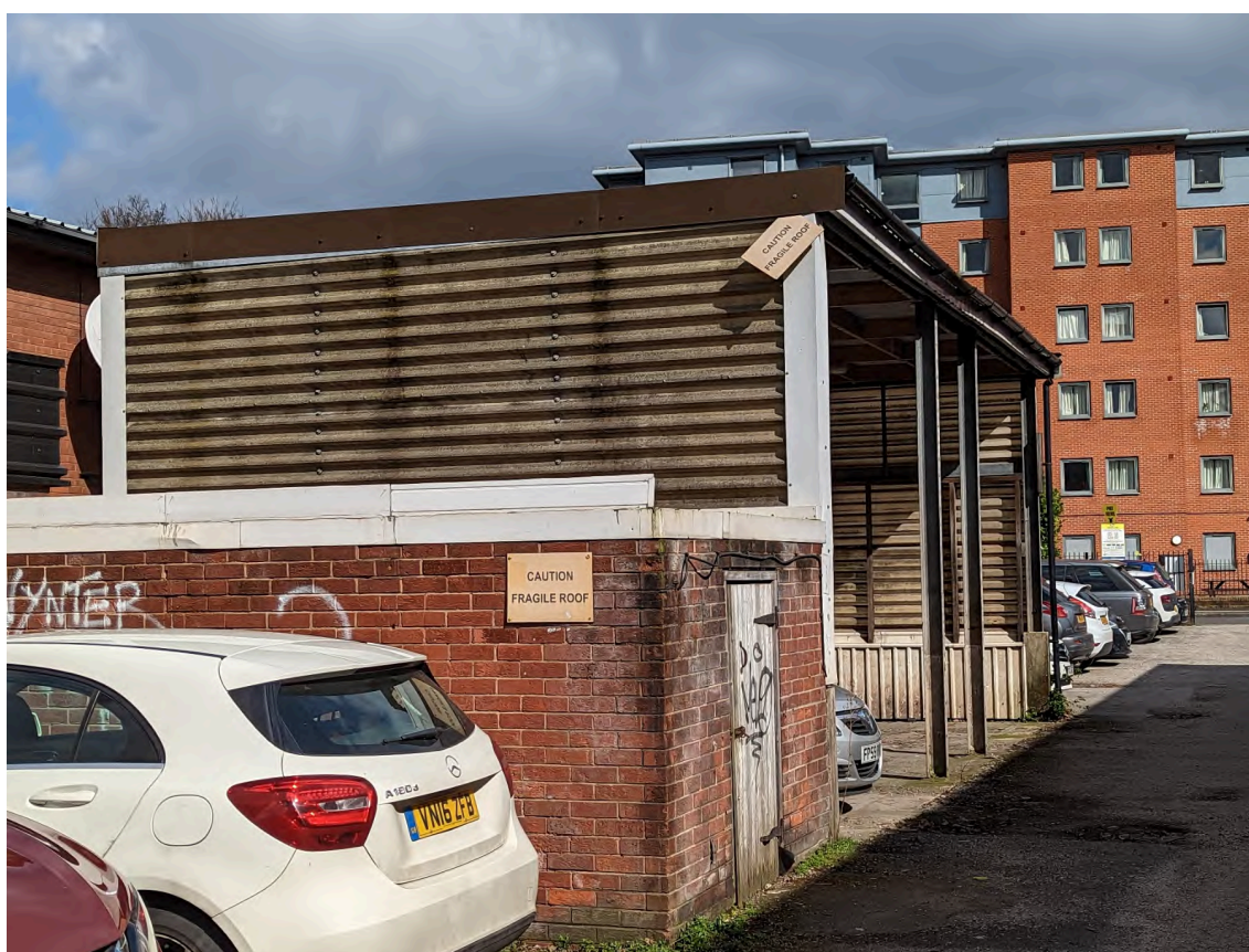
Image 8: Car store/wash area and non-accessible store with Fragile Roof caution signs
