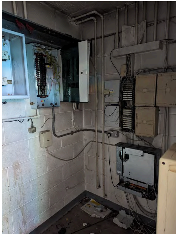
Image 2: Electrics and pipework servicing the car garage
