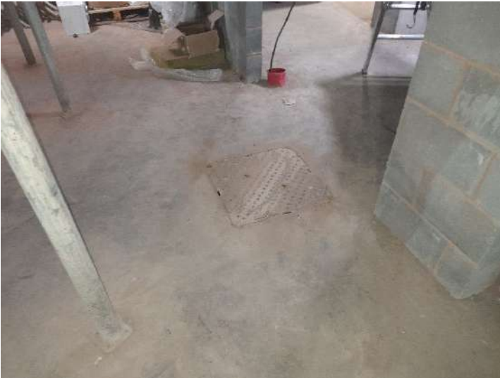
Photo 8 – FW08 Type B Manhole Cover
