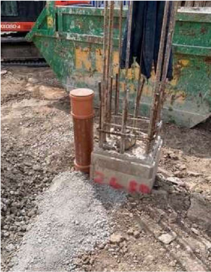
Photo 3 – Foul Pop-Up Adjacent Structural Columns
