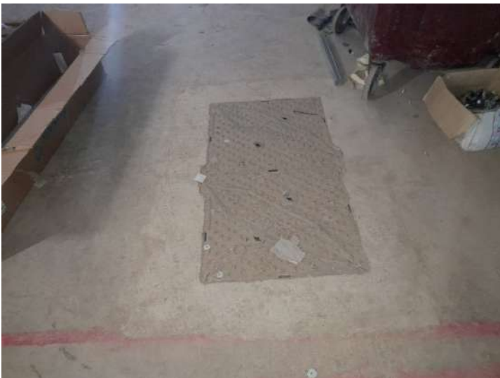
Photo 17 - FW04 Type C Manhole Cover
