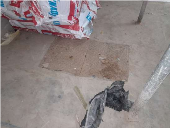
Photo 10 – FW07 – Type C Manhole Cover
