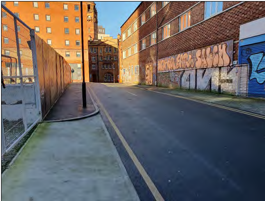
Photo plate 5. Echo Street. New footway surfacing on western side. Some uneven levels on eastern side.
