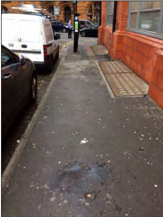
Photo plate 3. South Pump Street eastern footway. Adequate surfacing and width but pinchpoint created by street furniture.
