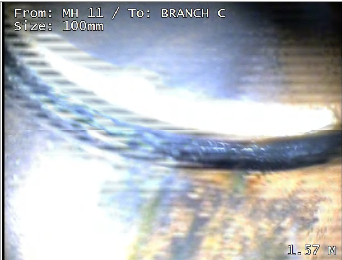
Line of drain/sewer deviates right
