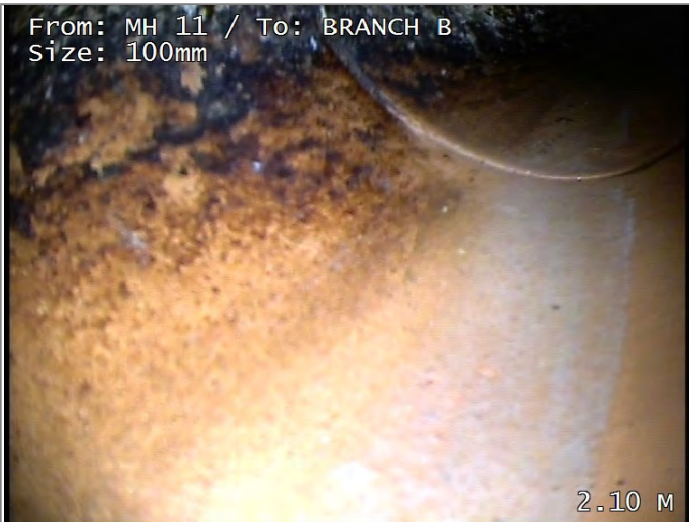
Line of drain/sewer deviates right
