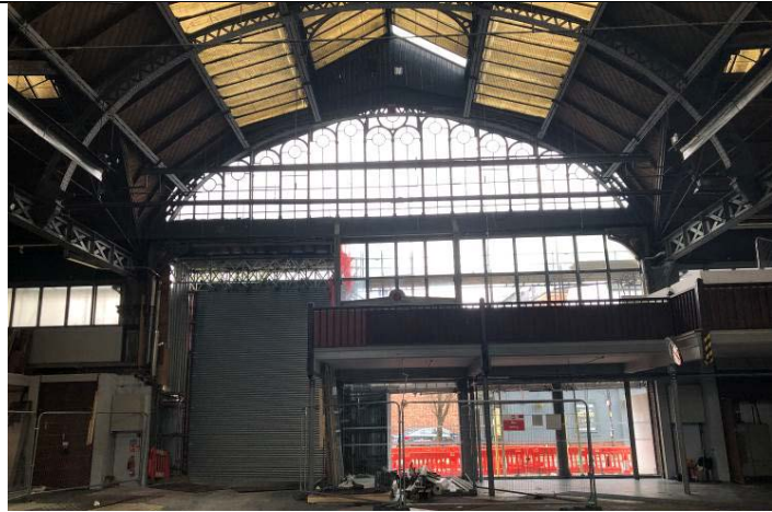
Figure 26: The central section of the south elevation, illustrating the discoloured 1980s roof coverings.
