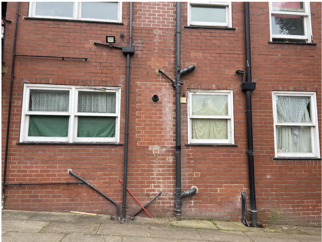
Rear elevations showing deterioration in the window frames and locations where previous windows were removed under the permission granted in 2018 (see below)
