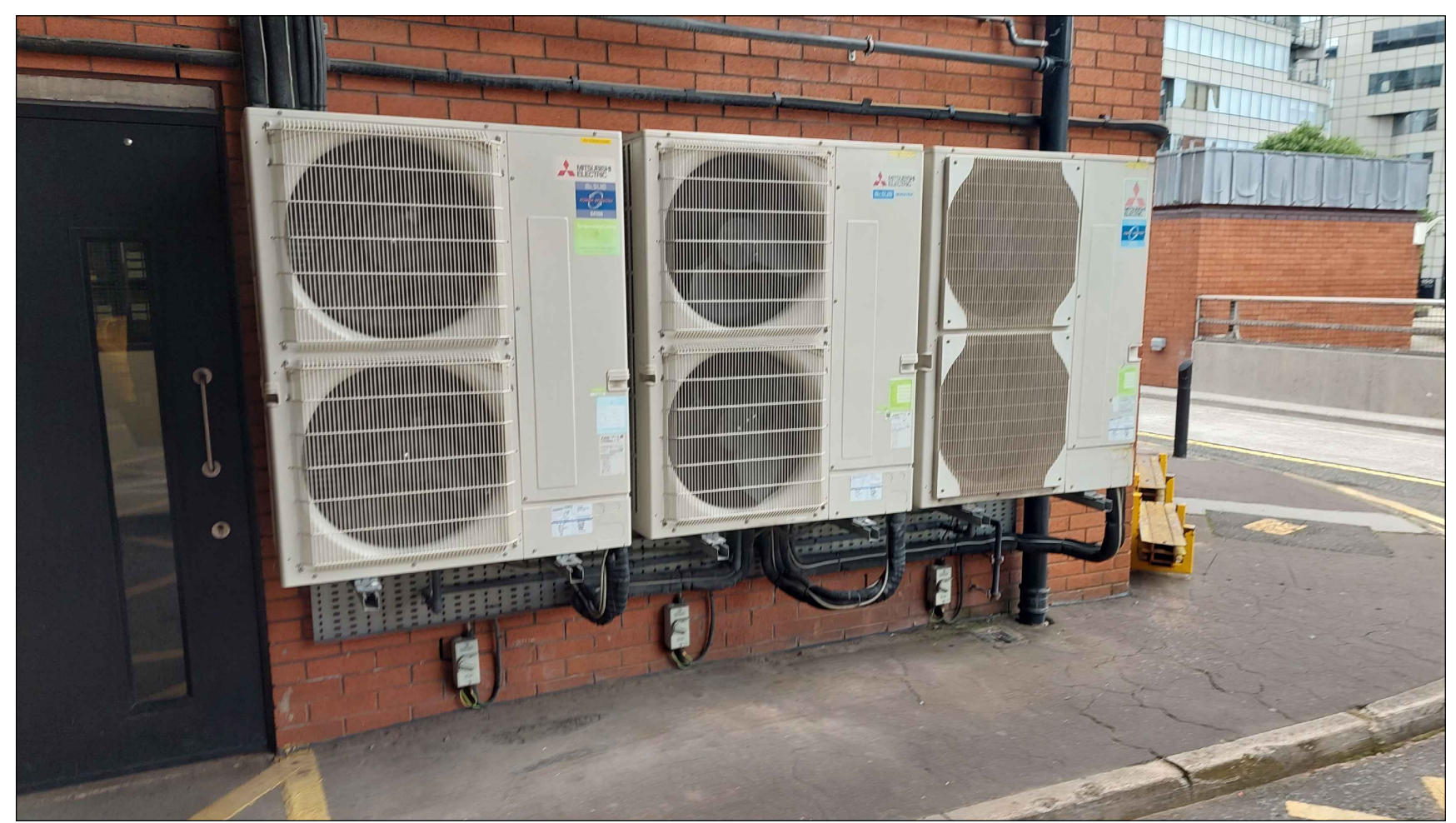
PHOTO 2 - EXISTING 3NO. CONDENSERS TO BE REPLACED FOR NEW. NEW SUPPORT FRAMES SHALL BE INSTALLED IN THE SAME POSITIONS AS EXISTING.
