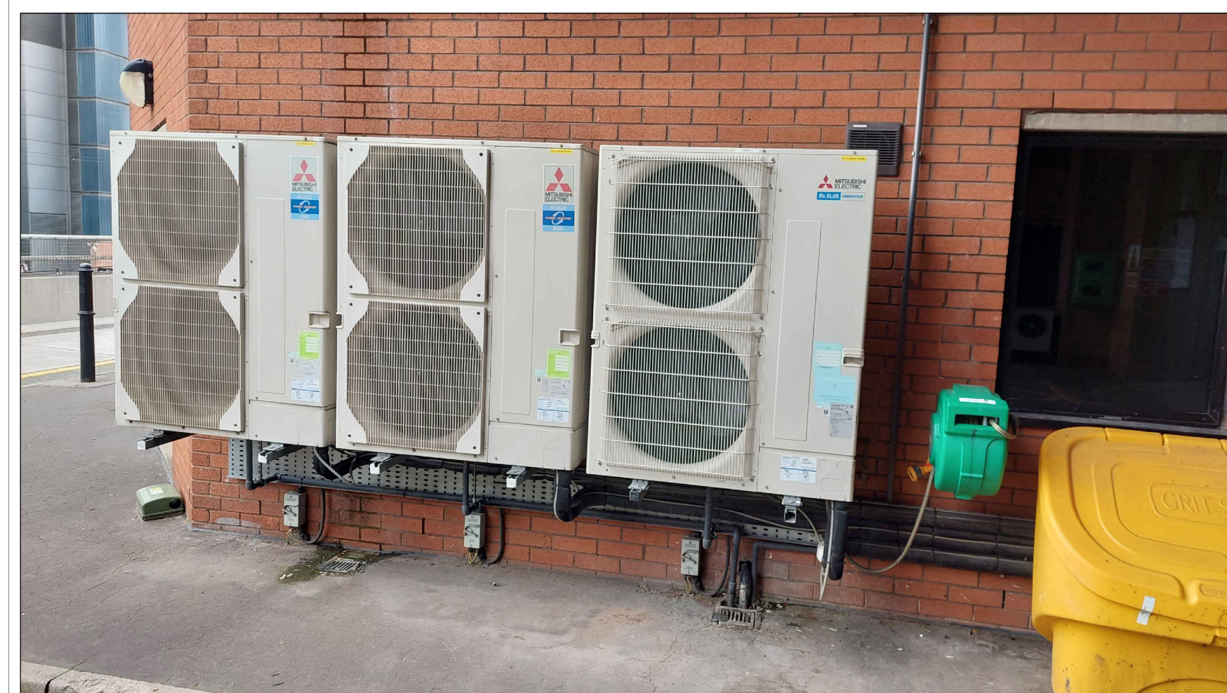
PHOTO 1 - EXISTING 3NO. CONDENSERS TO BE REPLACED FOR NEW. NEW SUPPORT FRAMES SHALL BE INSTALLED IN THE SAME POSITIONS AS EXISTING.
