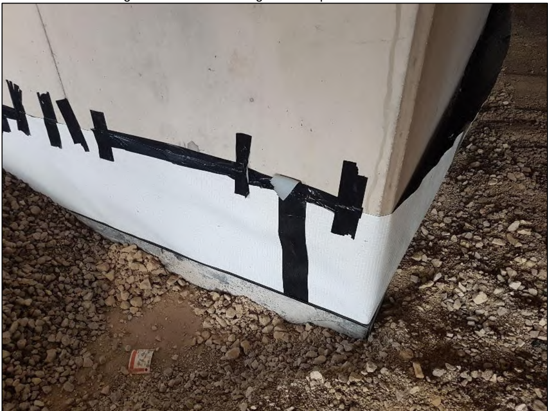
Figure 2: Photo showing southern area prior to installation
