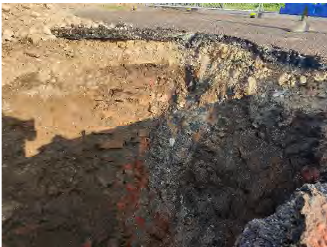
Photo No. 8: TPI04
